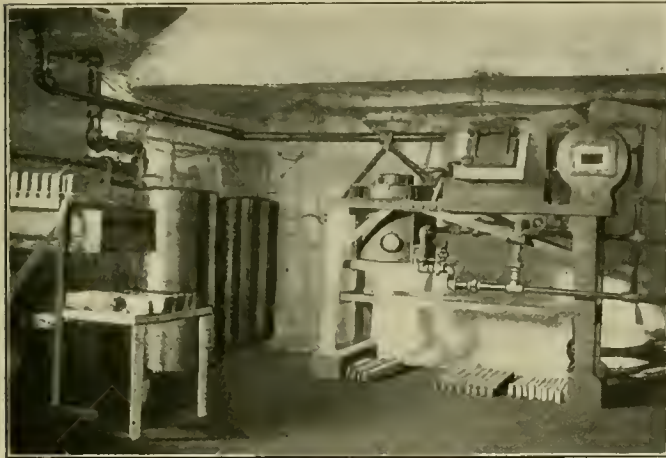
Fig. 17—Interior of Tempering Plant for a Small Shop
