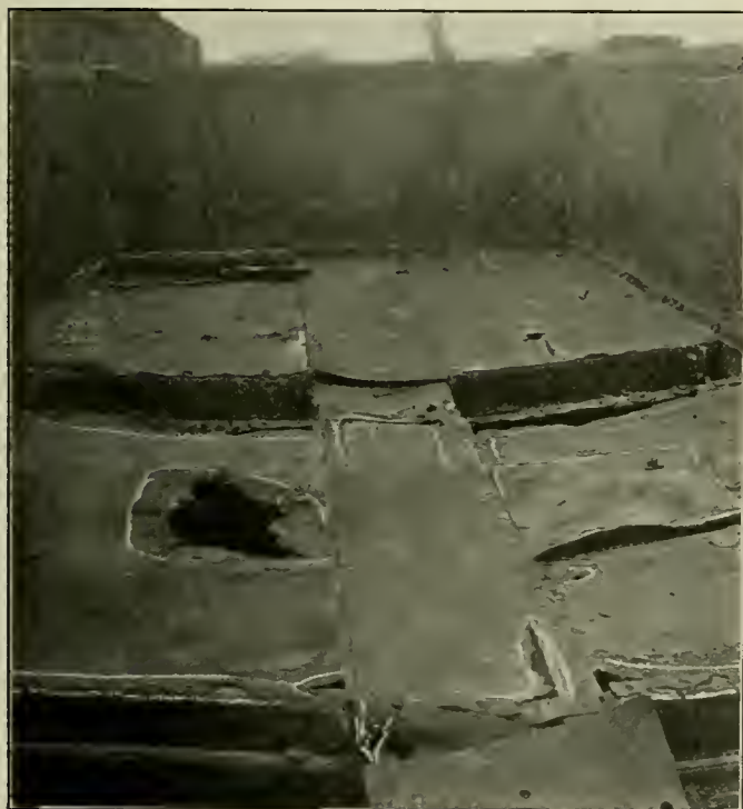
Fig. 7—A Drop Bottom Gondola with Floor and Sides Rusted so That no Sheets Were Fit for the Application of New Material
