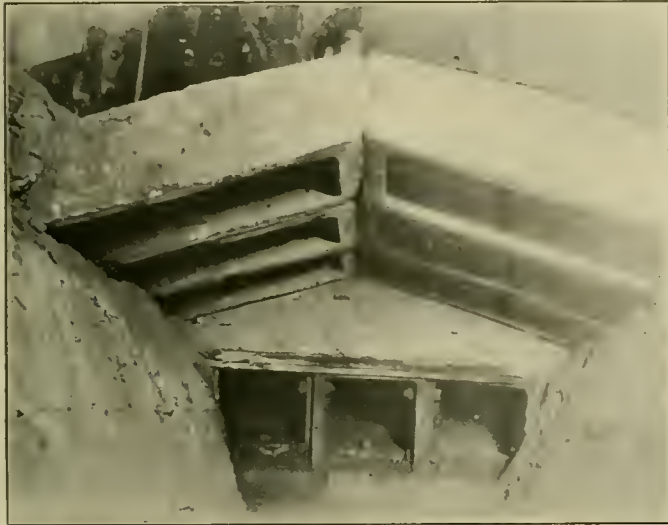
Looking Toward the Back of the Firebox, Showing the Primary Arch and the Burners
