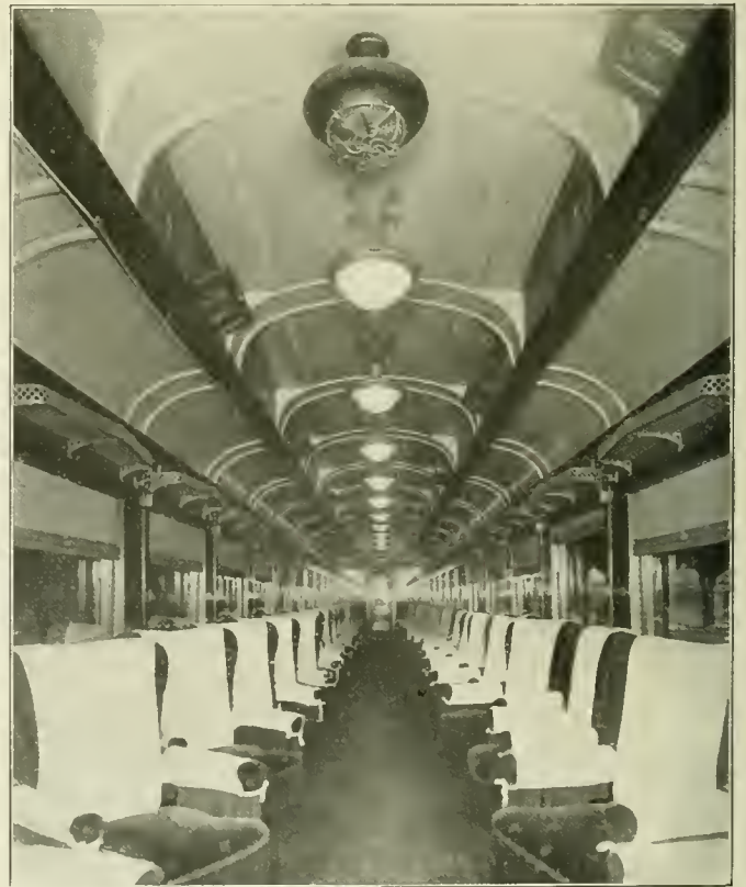
Application of the Indirect Fan to a Parlor Car; the Fans Are Placed Two Fixtures Apart
