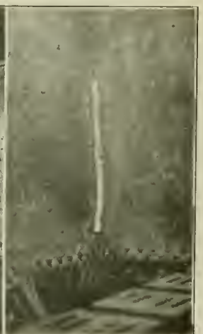
Fig. 5—Firebox Corner Weld
