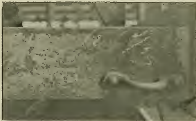
Fig. 12—Side Sill of a Steel Car Seven Years Old, Showing Corrosion Due to Lack of Paint
