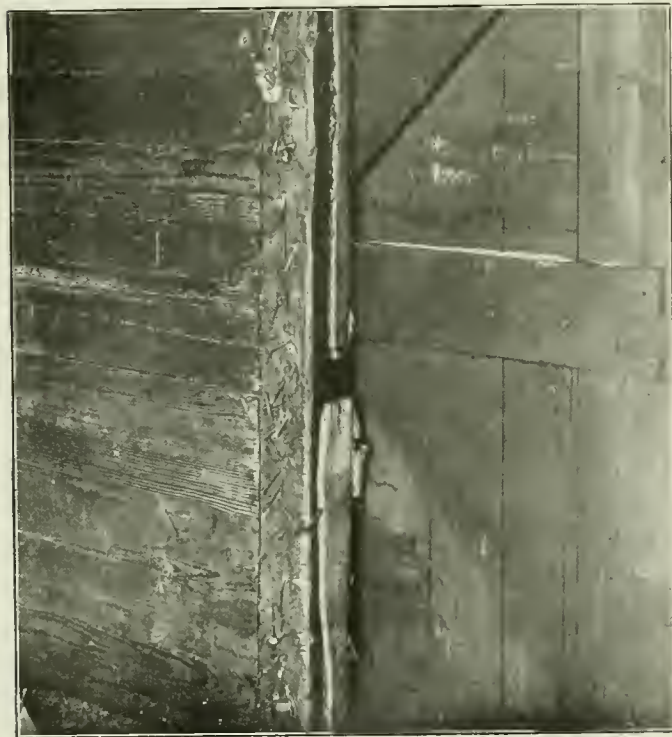
Door Post Damaged by Use of an Ordinary Type Grain Door
