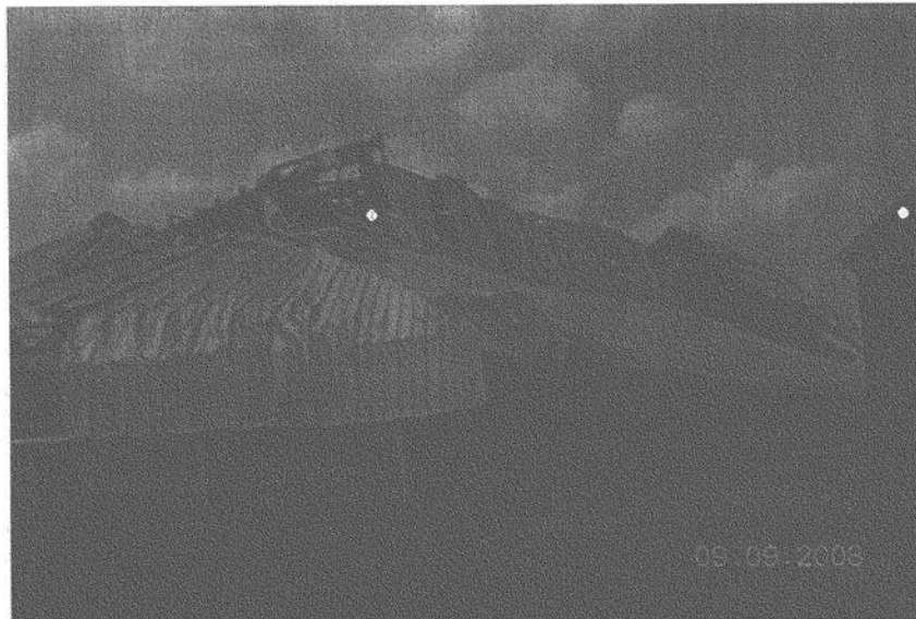
Raw Sugarcane Warehouse Damage
