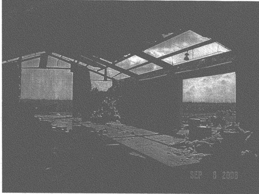
USDA Research Farm Equipment Maintenance Facility Damage
