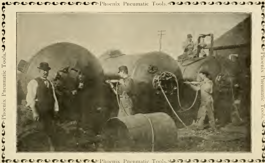
View taken at the Lebanon Boiler, Foundry and Machine Co.'s Works, at Lebanon, Pa., showing the utility of our Compressed Air Drills and Caulking Tools for outside work. Work shown was over 100 feet outside of boiler shop.
