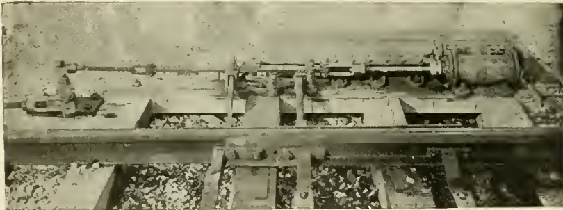
SWITCH OPERATING FOR THREE YEARS WITHOUT SINGLE FAILURE.
