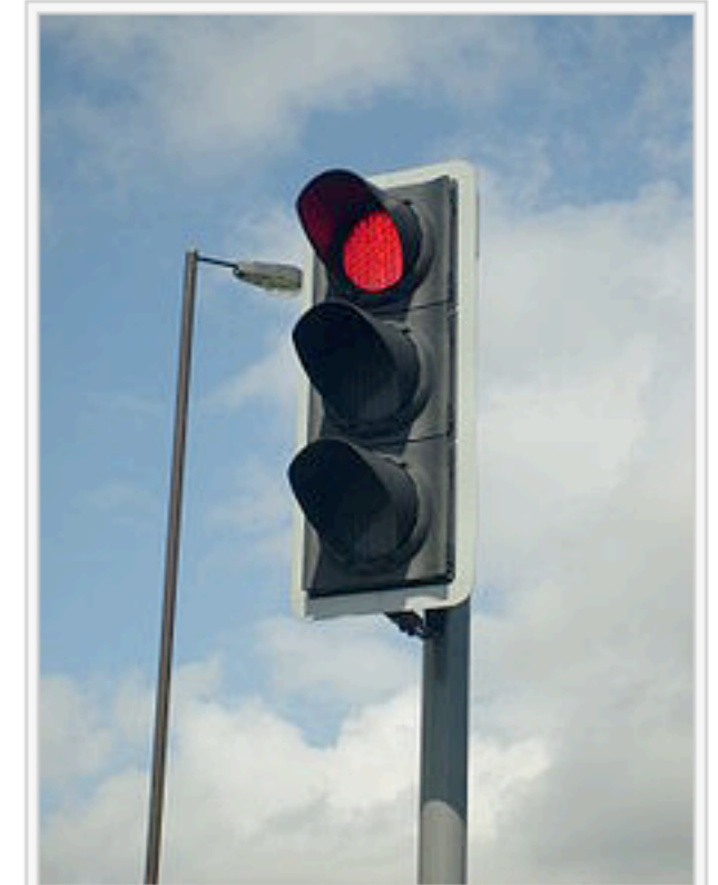
An LED traffic light in Portsmouth, England .
