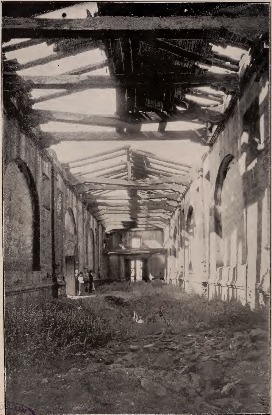
THE CHURCH AT SAN FERNANDO. (Since solidly re-roofed by the Landmarks Club.)
