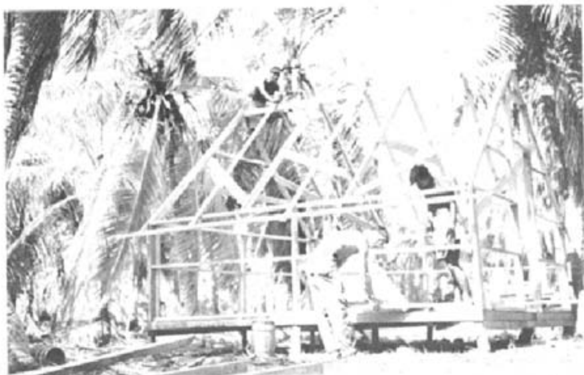
Figure 3. Navy Construction Battalion personnel, assisted by Marshallese, construct wooden house frames on Rongerik for Bikinians.
