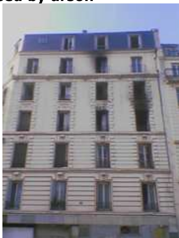
The building after the fire
