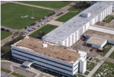
Damage at Stennis Space Center
