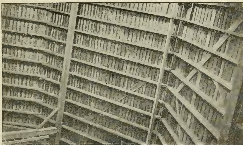
FIG. 341.—Method of trussing roof. Truss is 1 ft. by 8 in. hard wood let into upper surface of rafters and securely nailed to each rafter.
