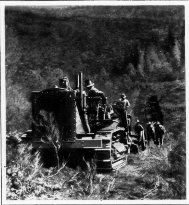
Cutting a Firebreak through Brush and Grass with the Big Tractor Outfit That Helps Protect California Forests
