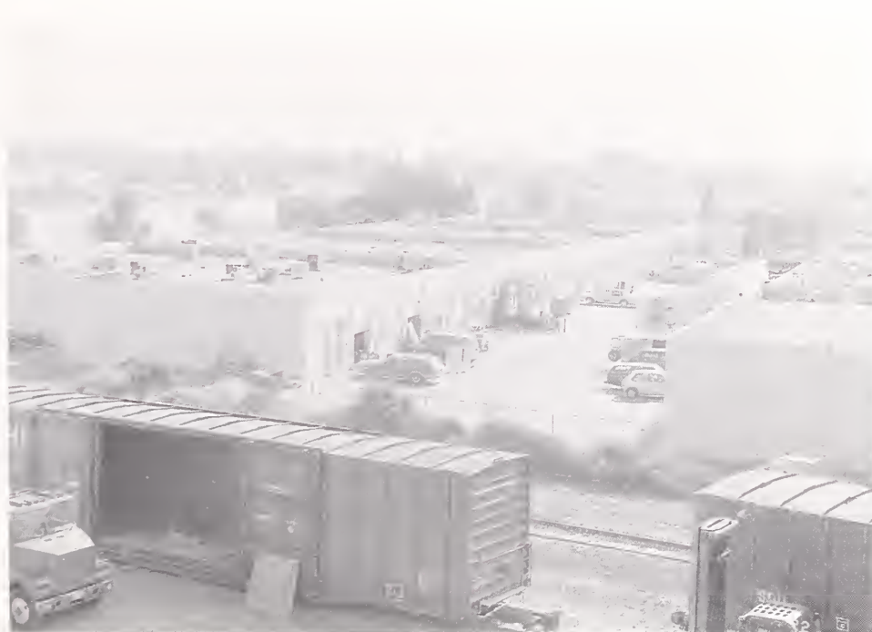
Figure 3.34. The single-story modern masonry commercial buildings directly south of the damaged Levitz furniture store and train derailment were apparently undamaged. All parapets and piers between garage openings appeared intact.
