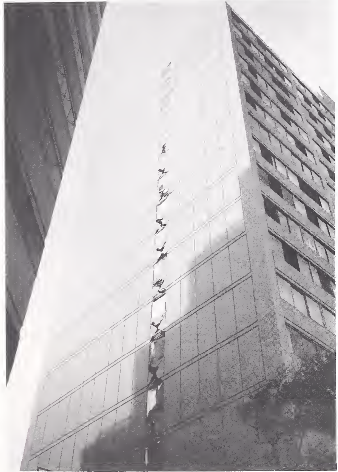
Figure 3.12. Champagne Towers apartment building in Santa Monica suffered a classic form of earthquake damage: shear failure of the coupling beams between linked shear walls at the transverse end of the building.
