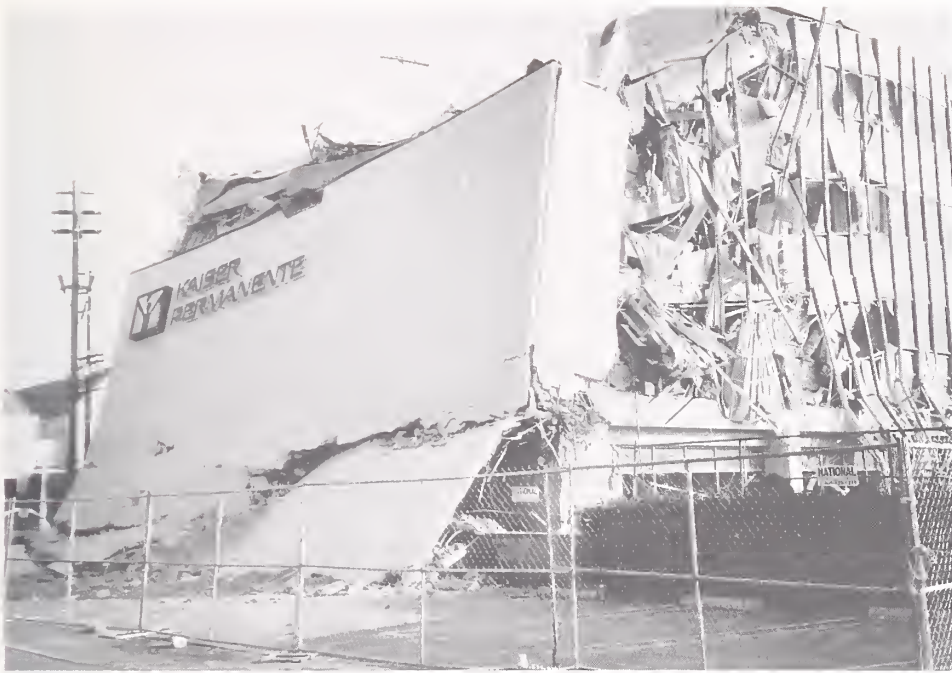
Figure 3.43. Damage at the north end of the building was similar to damage at the south.
