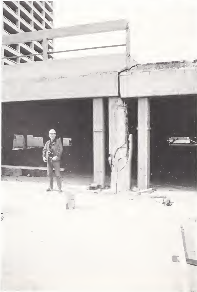
Figure 3.65. The exterior columns of the Trans World Bank parking garage, which had not been strengthened, were badly damaged.
