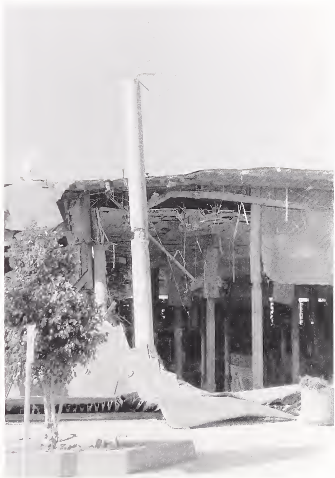
Figure 3.29. A portion of the concrete waffle slab roof and the interior floor slabs at the Bullock's department store at the Northridge Fashion Center mall fell to the basement, leaving many of the columns standing. No reinforcing steel can be seen in the remaining columns that would have connected the columns to the floor slabs.
