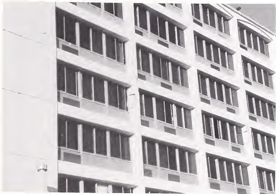
Figure 3.16. The bottom two stories of the concrete frame Holiday Inn in Van Nuys were damaged in the 1971 San Fernando quake and subsequently repaired. In the 1994 Northridge quake, damage was concentrated at the top of the fourth floor columns.
