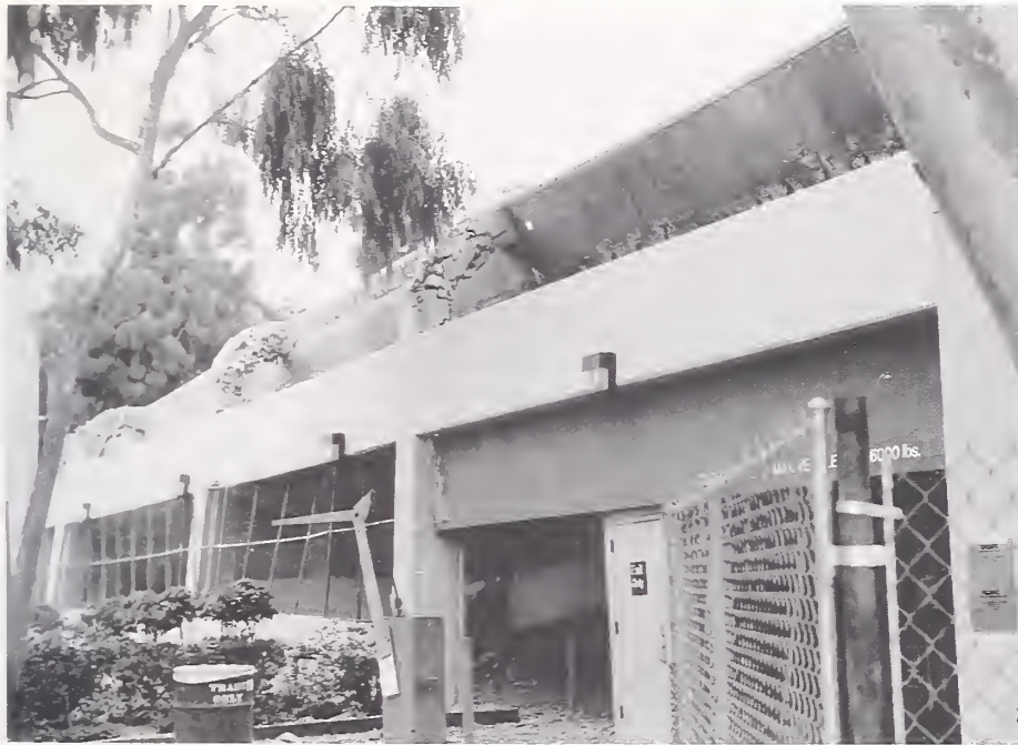
Figure 3.62. The cast-in-place concrete parking garage at the Kaiser Permanente Hospital complex in West Los Angeles collapsed in on itself. The moment frame that provided lateral resistance on the south face of the structure could not resist the out-of-plane forces apparently caused by the collapse of interior elements.
