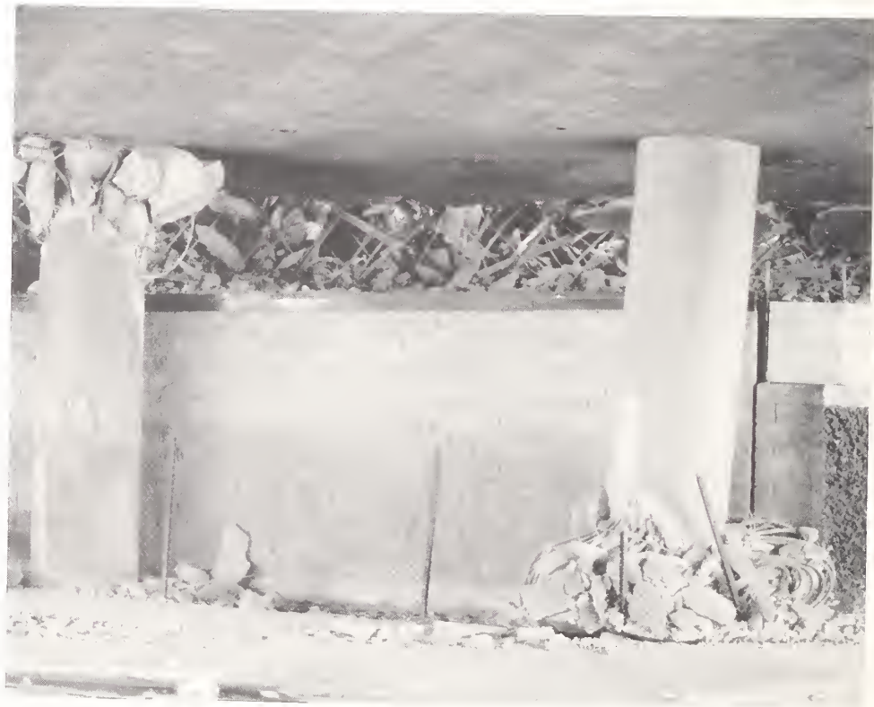
Figure 4.39. Failed piers in Bent 7 supporting westbound lane of I10 at Venice Blvd.
