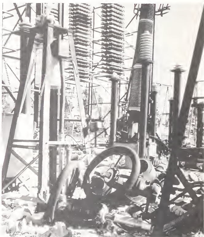
Figure 5.16. Porcelain is an integral part of high voltage electrical equipment due to insulation requirements and is also the most vulnerable to damage during strong earthquake shaking. (Photo courtesy of Edward Matsuda, Pacific Gas and Electric Company.)
