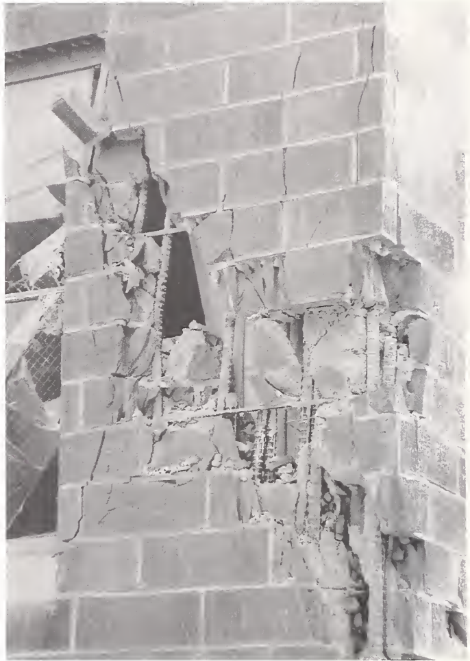
Figure 3.27. The facade of the five-story Berkley Convalescent Hospital directly adjacent to the St. John's Hospital complex consisted of two wythes of brick masonry with a reinforced and grouted space between. In some places, all three layers of this facade were destroyed along lines of diagonal cracking. The facility was evacuated.
