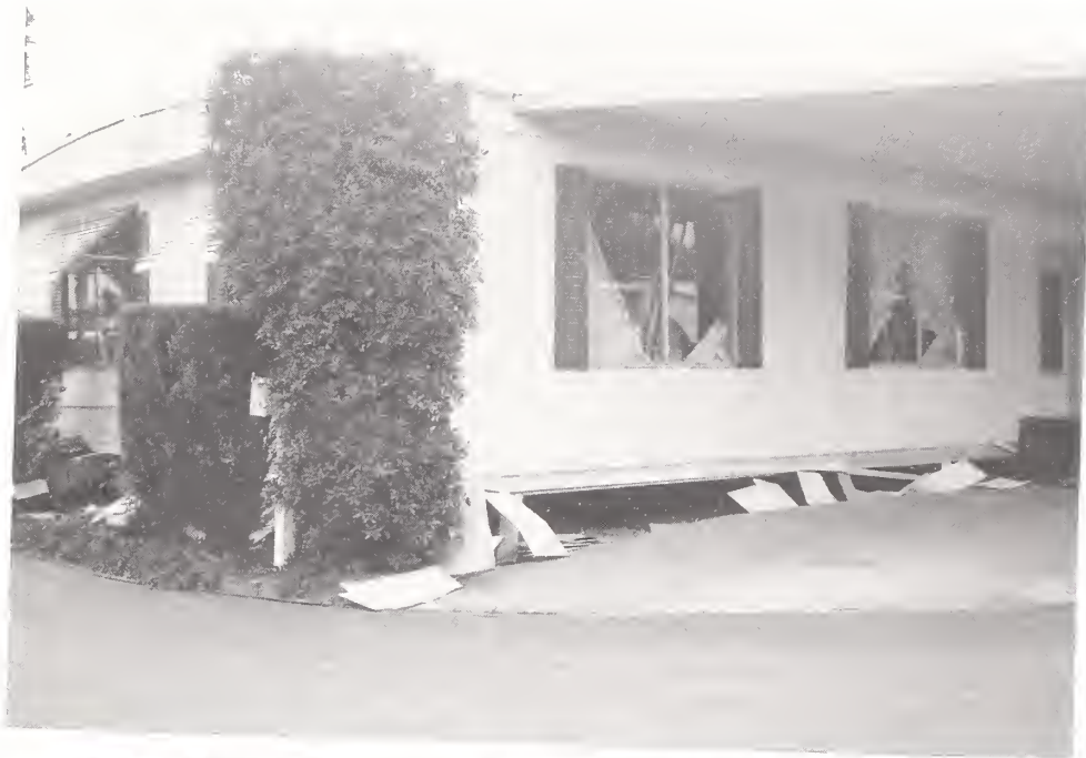
Figure 3.19. Damage to manufactured homes caused by collapsed supports was common.
