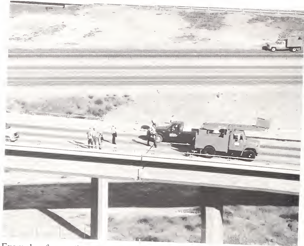
Figure 4.7. Example of pounding and offset at a hinge in the SR14/I5 interchange.
