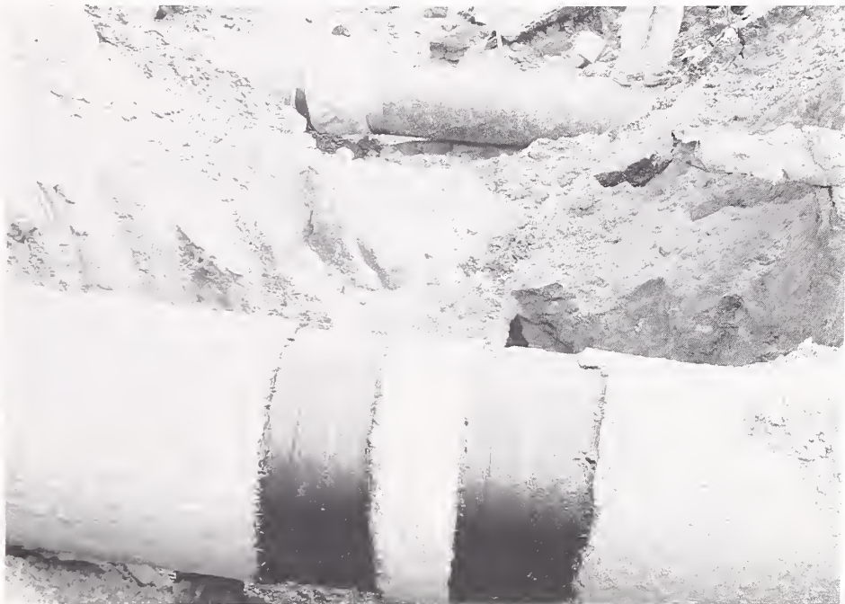
Figure 5.11. Ground extension along Balboa Boulevard resulted in the rupture of the same gas main shown in figure 5.10 (top) and a 1.2-m (48 in) water main (bottom). The rupture of the gas main here caused a major fire that engulfed five houses.
