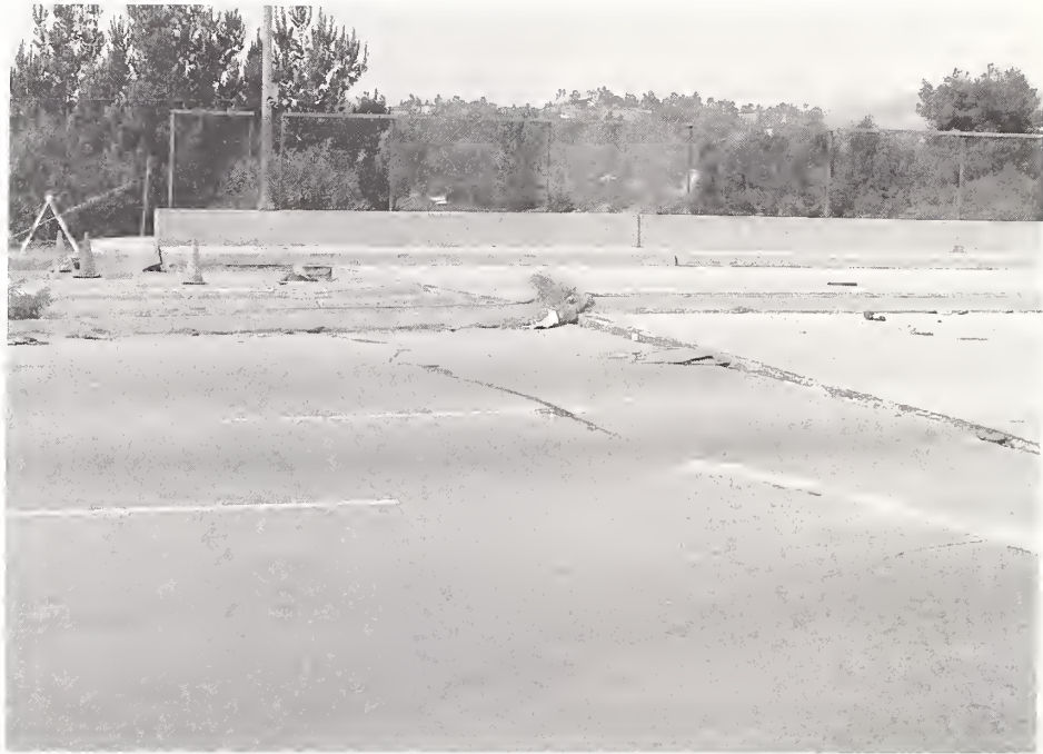
Figure 5.20. Transverse cracks in pavement near the intersection of Balboa Boulevard and SR118.
