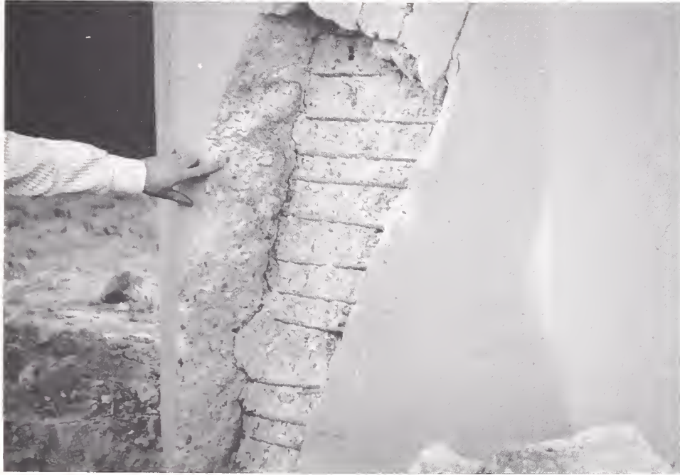
Figure 4.52. Close-up view of the westernmost pier at the Interstate 5, State Route 118, Southwest Connector, looking to the southeast. Loose cover concrete has been removed by Caltrans.
