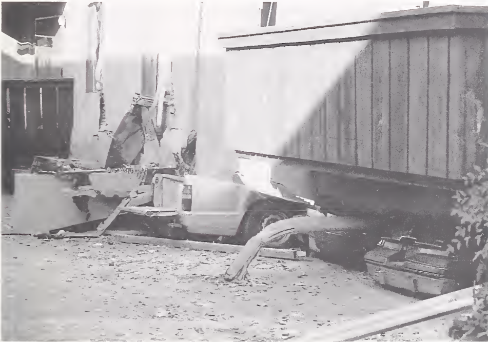
Figure 3.6. At Northridge Meadows, the first story steel pipe columns generally hinged near their bases but retained their length, controlling the displacement of the upper stories.
