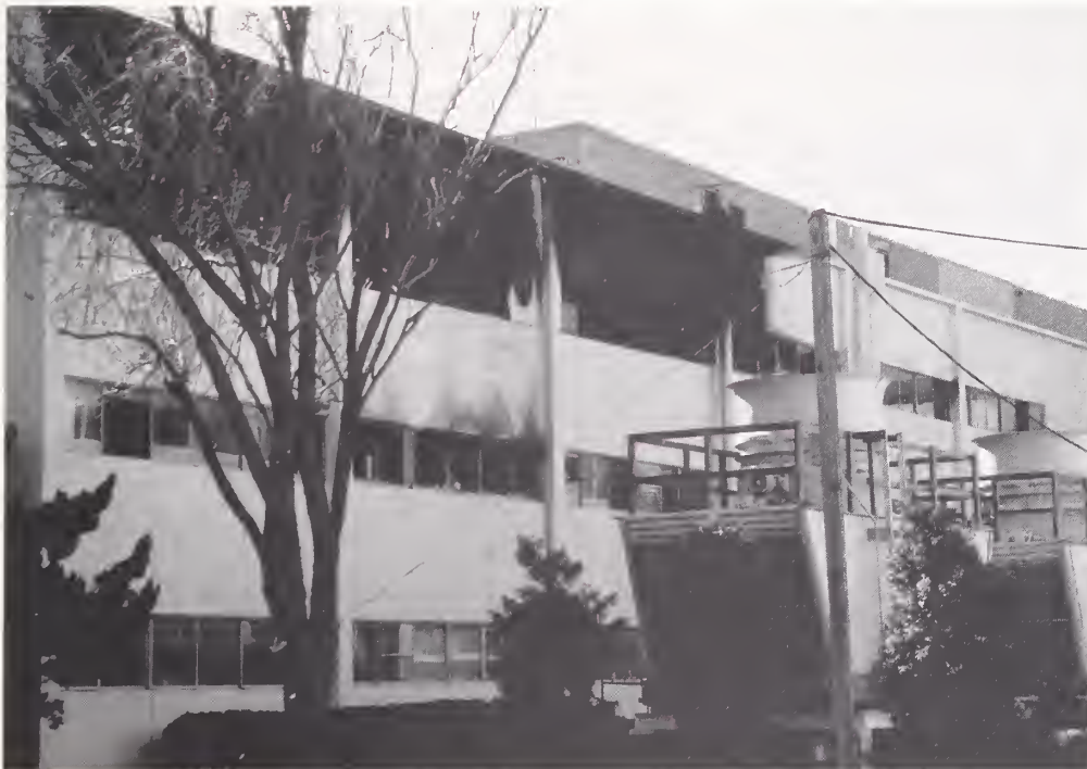
Figure 6.7. University science building damaged by fire.
