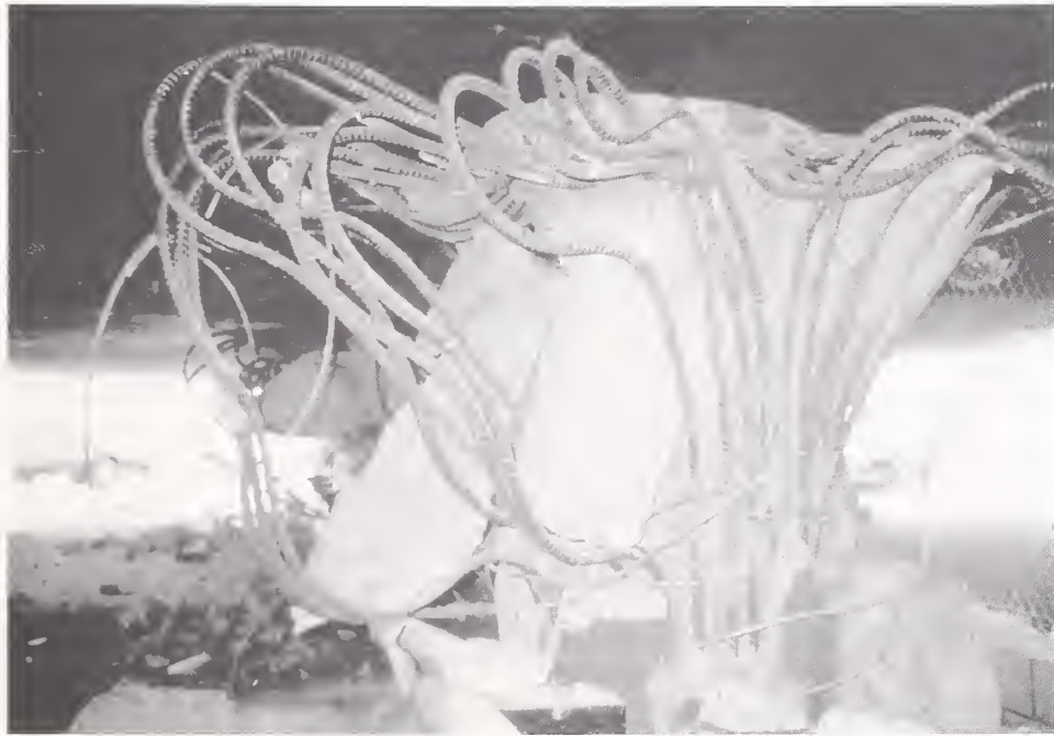
Figure 4.45. Failed column in Bent 3 of I10 at Fairfax Ave. (Photo courtesy of EERC).
