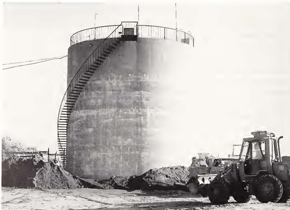
Figure 5.2. The reinforced concrete surge tank at Terminal Hill performed well during the earthquake--no damage was observed.
