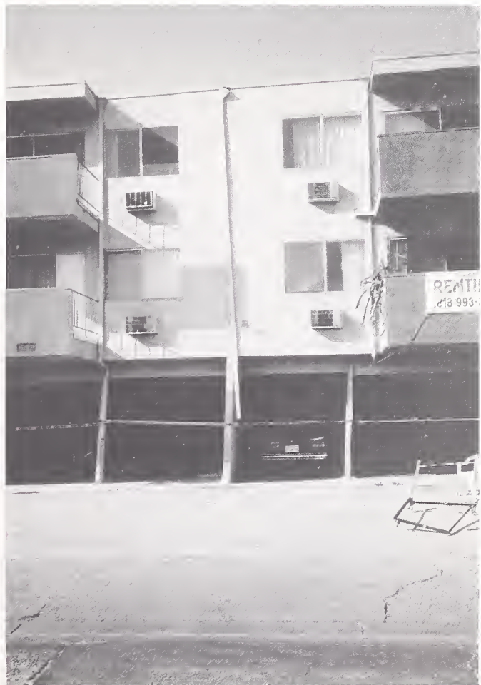
Figure 3.7. Racking, or leaning, of open first story parking areas was a common feature of damaged two and three-story apartment buildings.
