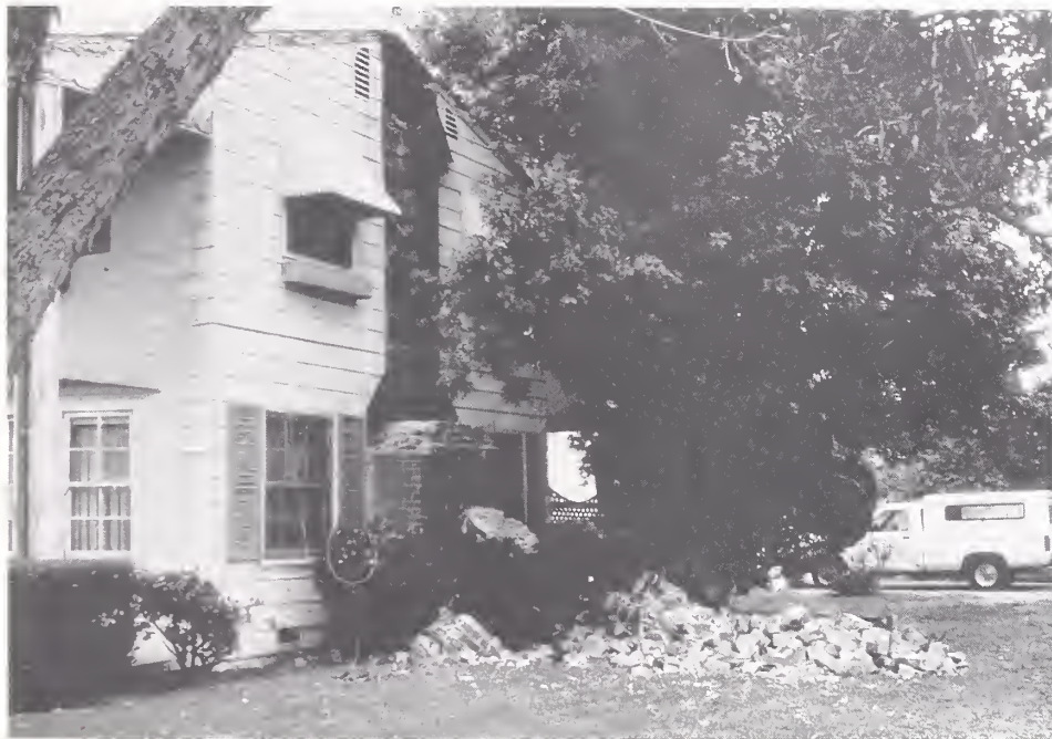
Figure 3.17. Failure of masonry chimneys was common.
