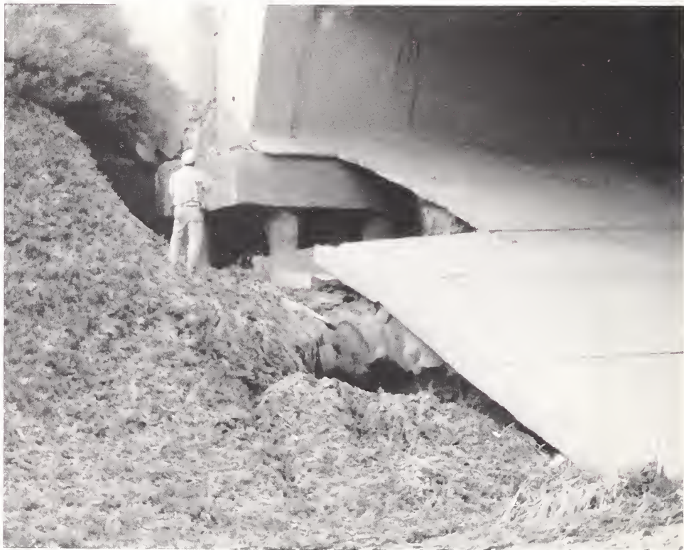
Figure 4.32. SR118 Balboa Avenue Overcrossing, view of the washout on the east side of the south abutment, caused by a ruptured water main.
