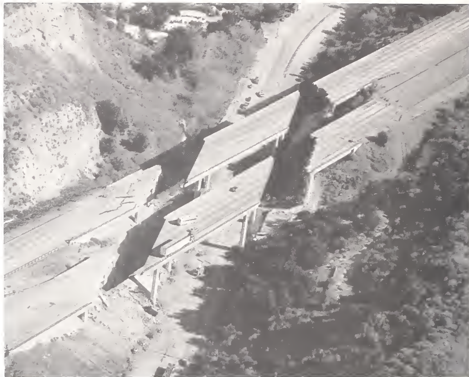
Figure 4.2. Aerial view of the bridges at Gavin Canyon, looking to the east, showing appearance of the four end spans shortly after demolition had begun.
