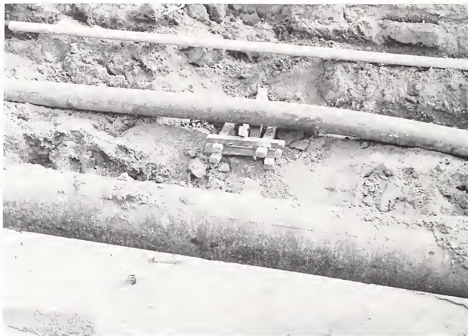
Figure 5.14. Some of the buried pipelines located near the intersection of Balboa Boulevard and Bircher Street showing the potential hazard of co-location of lifeline systems. At this site are three water lines (two of them main lines); three gas lines; two sewers; one crude oil line; overhead power, telephone, and cable TV lines; the street lighting system; and the street itself.
