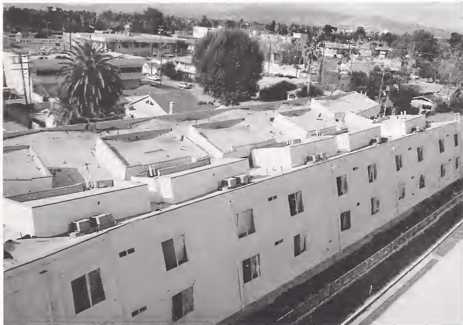
Figure 3.11. This overhead view of the partially-collapsed apartment building on Sherman Way shows the solid concrete masonry block perimeter walls along the longitudinal axis of the building. Access to the first story parking was limited to the transverse ends of the building. When the row of interior columns failed, both sides of the building settled in towards the middle.
