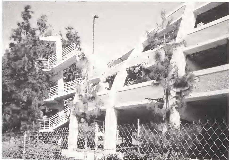
Figure 3.60. The three-year old four-level parking garage at the Northridge campus of California State University partially collapsed in the earthquake. The collapse apparently started at the interior, causing the exterior frame to be pulled in to the middle of the structure. Precast concrete "trees" were connected to form a moment-resisting frame at the exterior of the structure.
