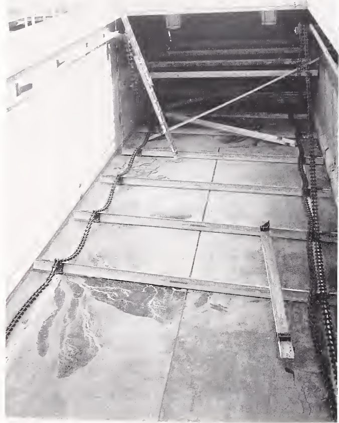
Figure 5.7. A damaged sludge scraper in a clarifier tank at the Tillman Water Reclamation Plant.
