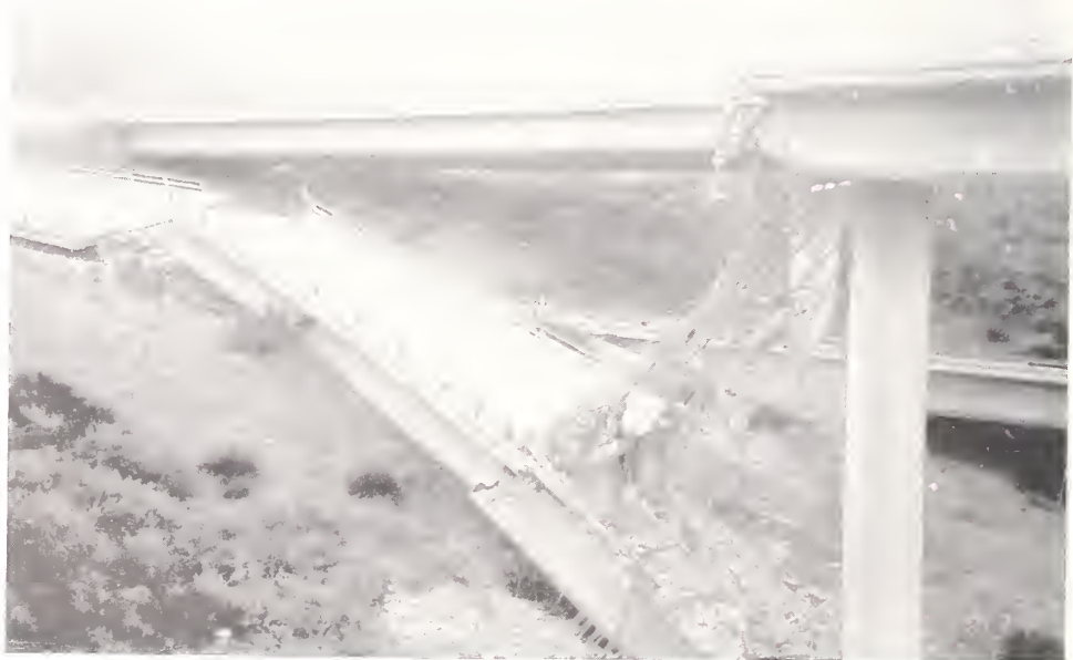
Figure 4.14. Collapsed portion of the SR14/I5 North Connector Overcrossing, looking east. Pier 2 was at the left, near the broken hinge on the ground (Photo courtesy of EERC).
