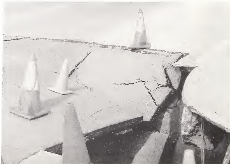
Figure 5.21. The approach of Balboa Boulevard at SR118 caved in due to the loss of the abutment fill because of a water main break.
