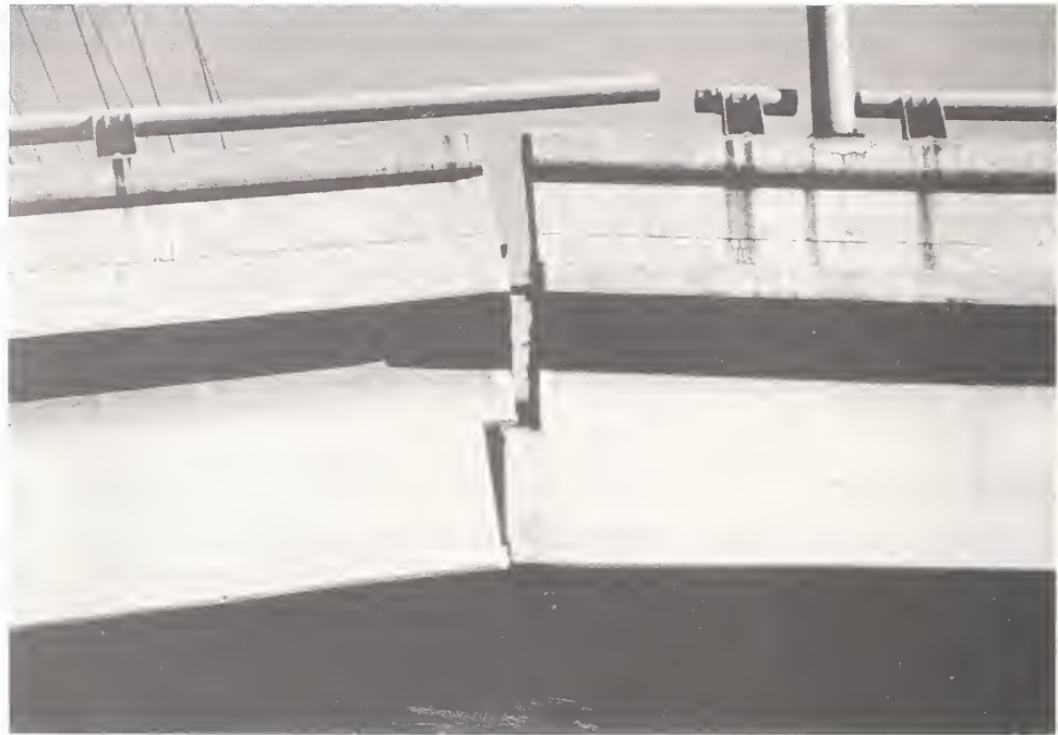
Figure 4.43. Hinge adjacent to Bent 4 of I 10 at Fairfax Ave.; cable restrainers prevented loss of support (Photo courtesy of EERC).
