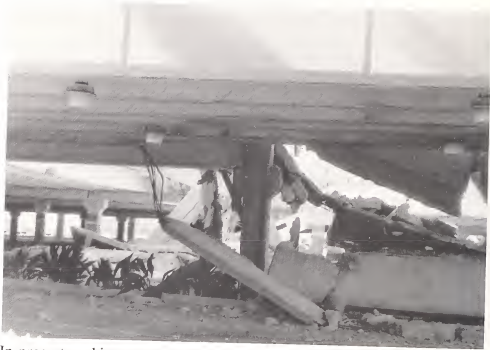
Figure 3.68. In precast parking garages, the support of the double-tees that comprise the floors is a vulnerable link in the system. This garage, at the north end of the Northridge Fashion Center, illustrates a common failure: the double-tees pulled off their supports, leaving the supporting elements essentially intact.
