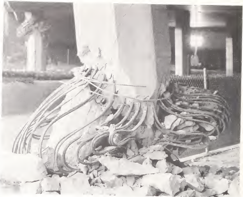
Figure 4.27. Damage to pier 3S-1 of State Route 118 at Bull Creek Canyon Channel, looking to the northwest.
