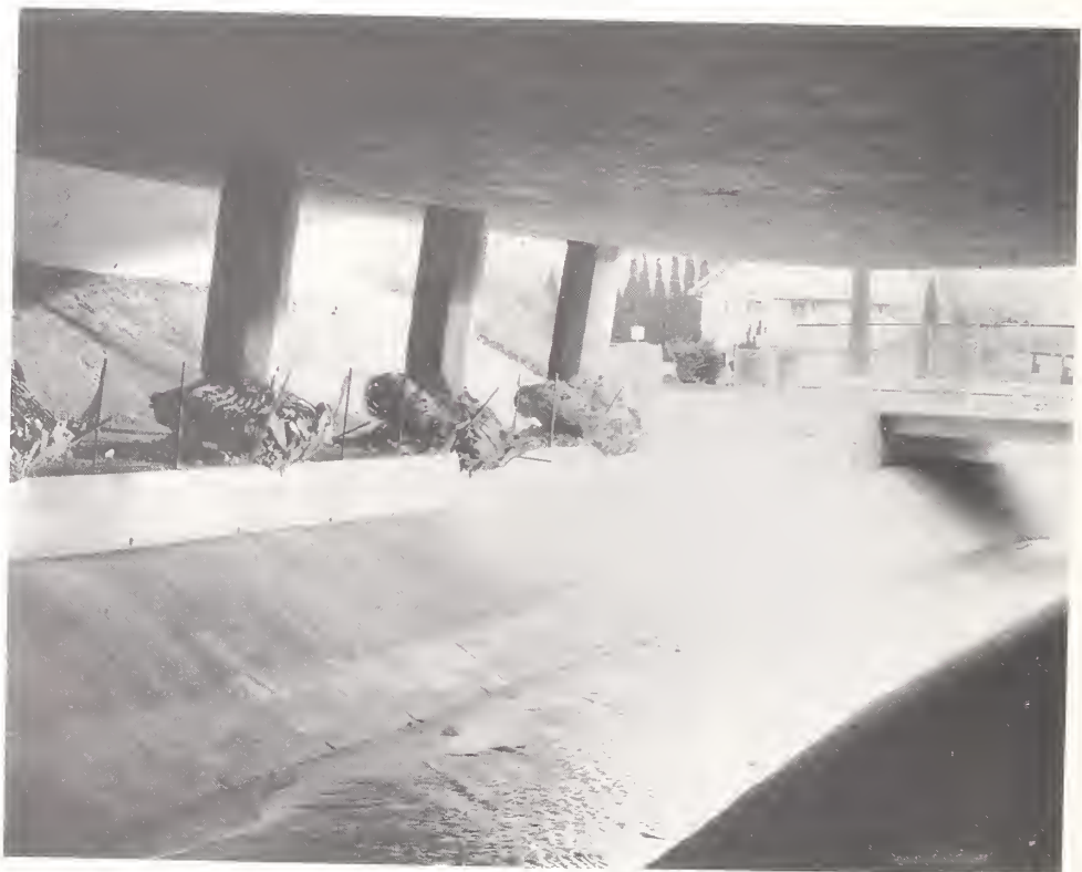
Figure 4.28. Damage to piers of Bent 3S of State Route 118 at Bull Creek Canyon Channel, looking to the southeast.
