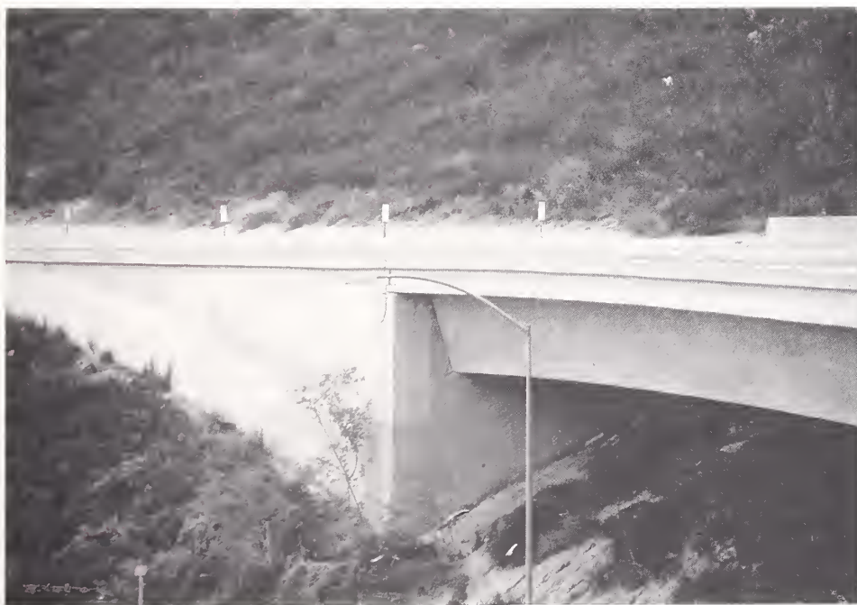
Figure 4.56. Overview of abutment at the east end of the ramp connecting eastbound SR118 with northbound I210.
