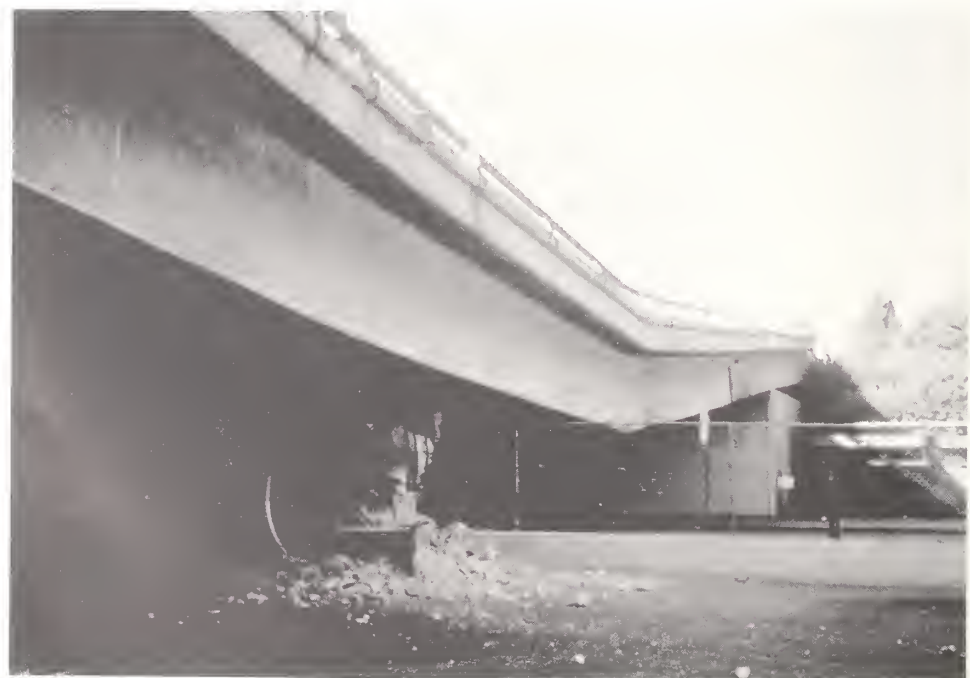
Figure 4.44. View of collapsed span of I10 over Fairfax Ave.; note rotation of girder over Pier 2 (Photo courtesy of EERC).
