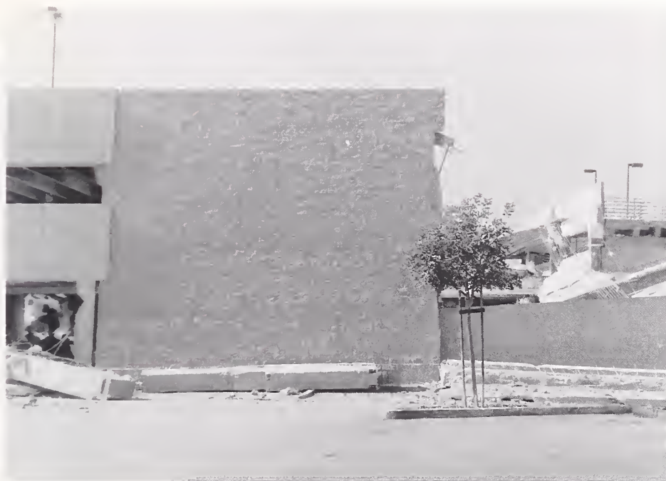
Figure 3.66. At the Northridge Fashion Center, major portions of the three-level south parking garage collapsed. The garage was precast concrete with intermittent shear walls. Most of the shear walls remained standing, largely undamaged, indicating that the lateral load was not adequately transmitted to these walls.
