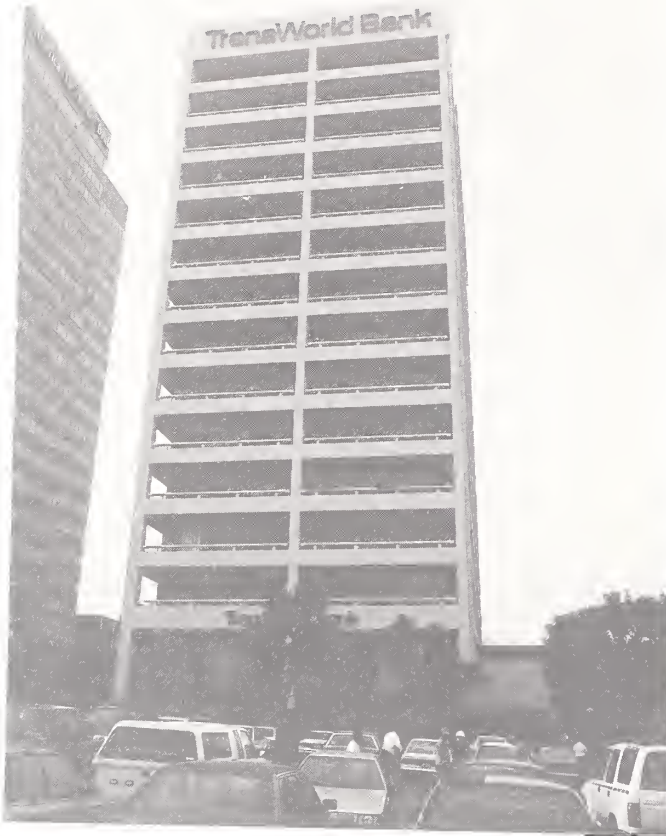
Figure 3.53. The Trans World Bank building, in Sherman Oaks, was damaged in both the 1971 San Fernando and 1994 Northridge earthquakes.
