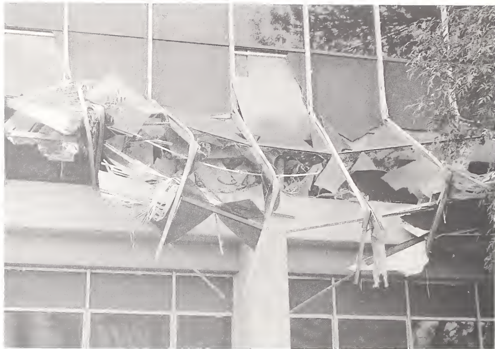
Figure 3.41. The second story of the concrete frame Kaiser Permanente office building on Balboa Avenue in Granada Hills completely collapsed. The first story was relatively undamaged, suggesting it was far stiffer than the story above.
