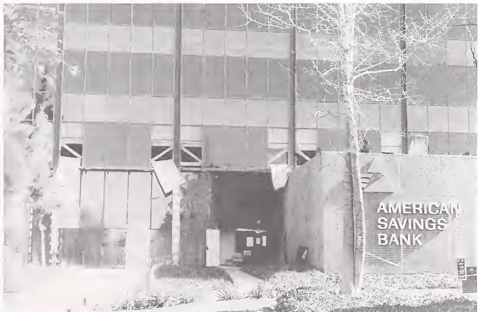
Figure 3.52. The first-story columns of the steel-framed building housing the American Savings Bank on Topanga Canyon Road in Canoga Park flexed during the quake and ended up slightly displaced from their original positions.
