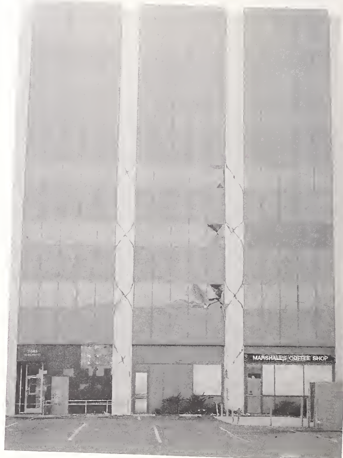
Figure 3.46. The stiff infill panels of the Barrington Building effectively shortened the concrete columns, forcing all the displacement into the column sections bounded by windows. Diagonal X-cracking decreased in severity towards the top of the building.
