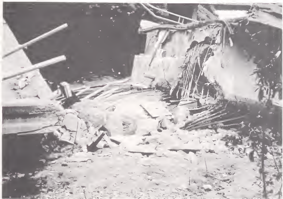
Figure 4.16. View of crushed Pier 2 and the hinge near Pier 2 (Photo courtesy EERC).
