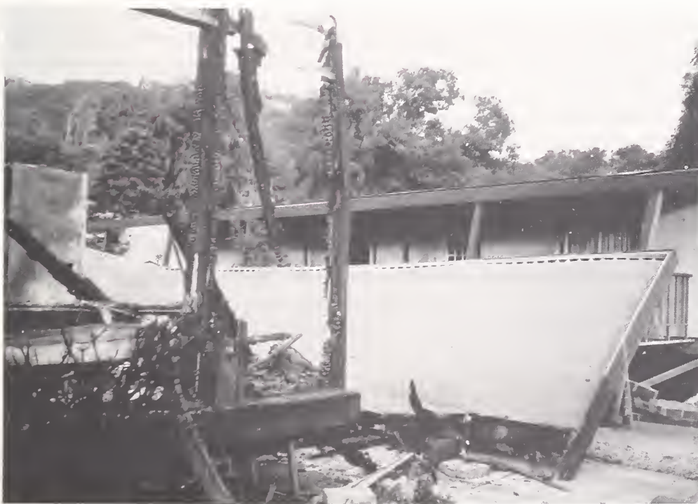
Figure 6.10. Collapsed roof which acted as a fire break in a manufactured housing development.
