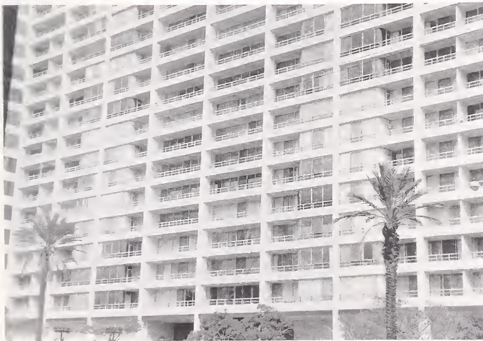
Figure 3.13. The front of the 16-story Champagne Towers building had no apparent damage. Note the steel pipe railings at the balconies.
