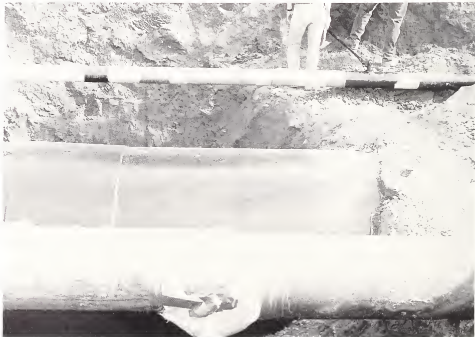
Figure 5.10. Ground contraction along Balboa Boulevard caused the rupture of a gas distribution line (top), the Rinaldi trunk 1.8-m (68 in) water main (center), and a gas main (bottom). The pipes were being repaired at the time this photograph was taken.
