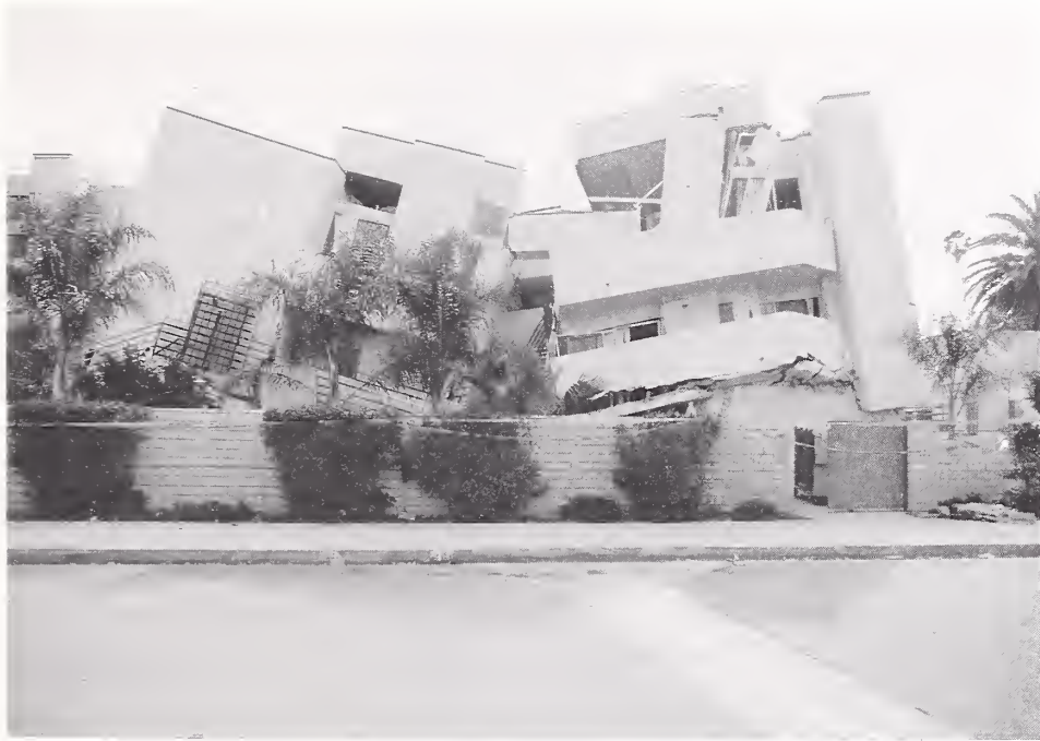
Figure 3.10. The central row of concrete first-story columns in a three story apartment building on Sherman Way in Van Nuys collapsed, causing the wood-framed upper stories to settle inward.
