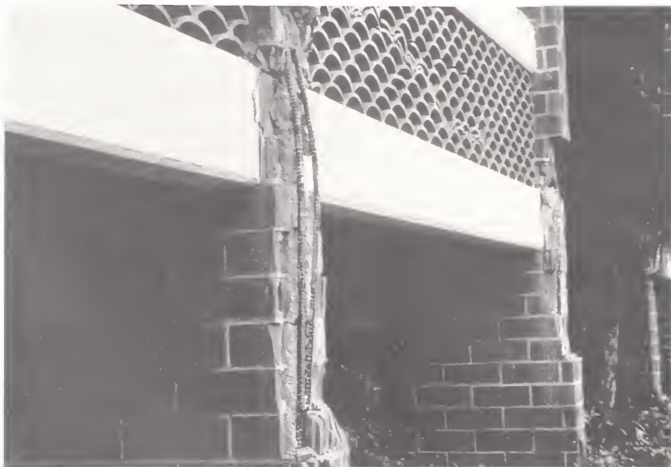
Figure 3.28. Two faces of the Berkley Convalescent Hospital had wing walls separating balconies. The ends of these wing walls spalled at the lower stories.
