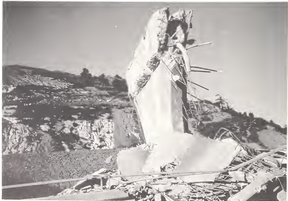
Figure 4.12. Damage at Pier 3 of the SR14/I5 Separation and Overhead, Ramp C, looking to the west (Photo courtesy of EERC).
