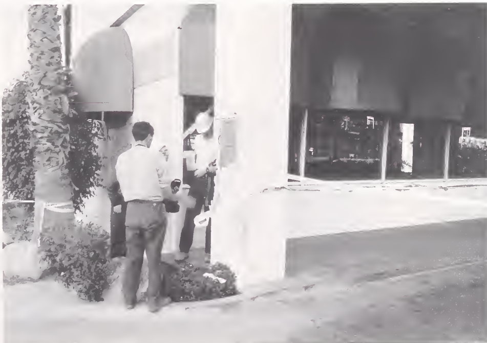
Figure 3.56. The columns supporting the three-story appendage at the front of the Radisson Hotel had serious shear cracks and related spalling.
