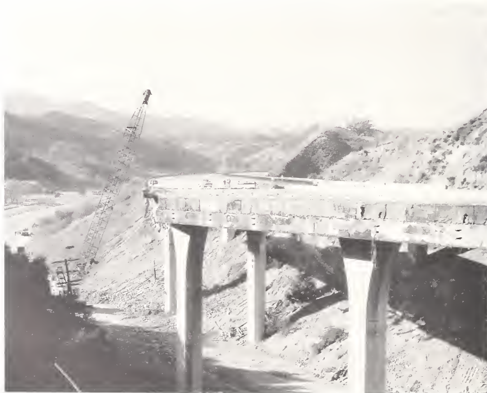
Figure 4.3. Ground level view of the southbound bridge at Gavin Canyon, looking to the northwest, showing the hinge bearing seat near Bent 3.
