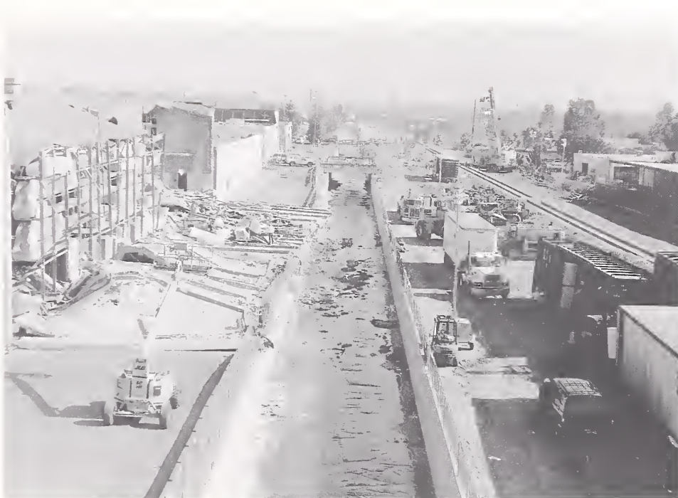
Figure 3.33. The south wall of the concrete tilt-up Levitz furniture store/warehouse south of the Northridge Fashion Center fell away from the building into the alley and stream channel. The damaged roof was being supported by the racks of furniture. On the south side of the stream channel a freight train derailed during the earthquake. That clean-up effort was still underway three days after the quake.
