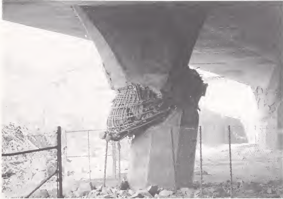
Figure 4.21. Damage to a pier of the SR118 Mission-Gothic Undercrossing, looking to the northwest at the southernmost pier of Bent 3 of the westbound bridge.
