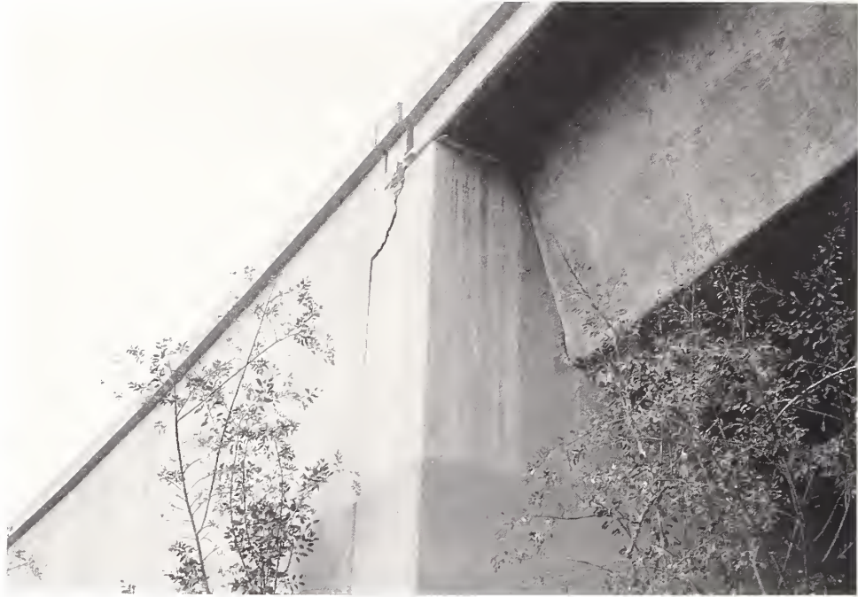
Figure 4.57. Close-up of abutment wall cracking at the east end of the ramp connecting eastbound SR118 with northbound I210.
