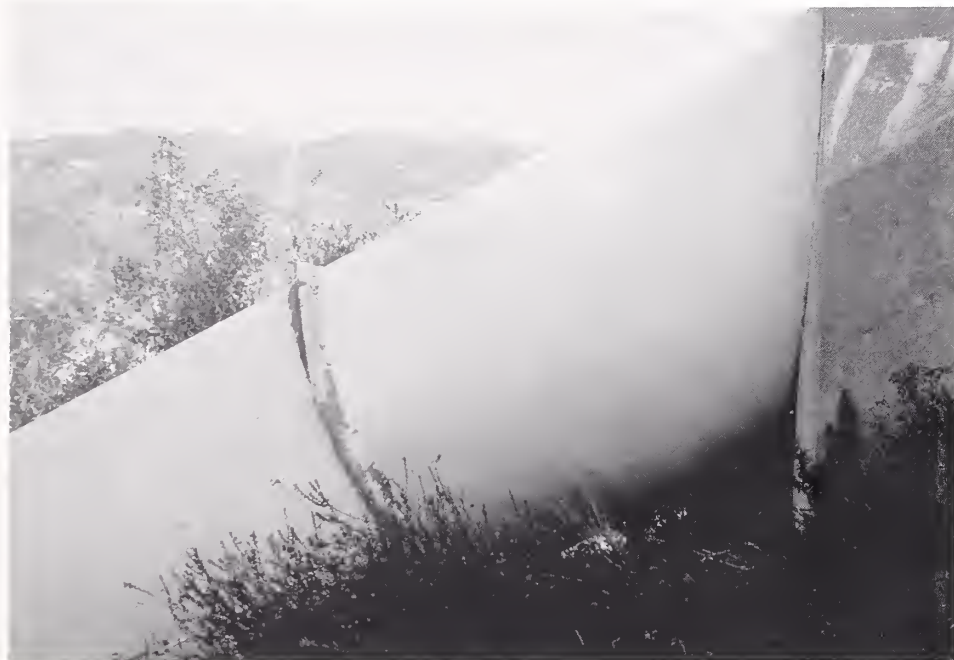
Figure 5.3. The steel pipeline at Terminal Hill separated from its supporting saddle at several places and pipe sections bulged at other locations along the alignment.
