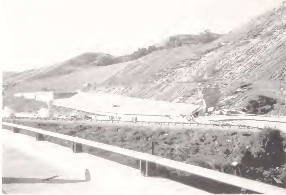
Figure 4.11. Overview of the collapse of the SR14/I5 Separation and Overhead, Ramp C, looking to the south at Abutment 1. Pier 3 can be seen at the right of the photograph (Photo courtesy of EERC).
