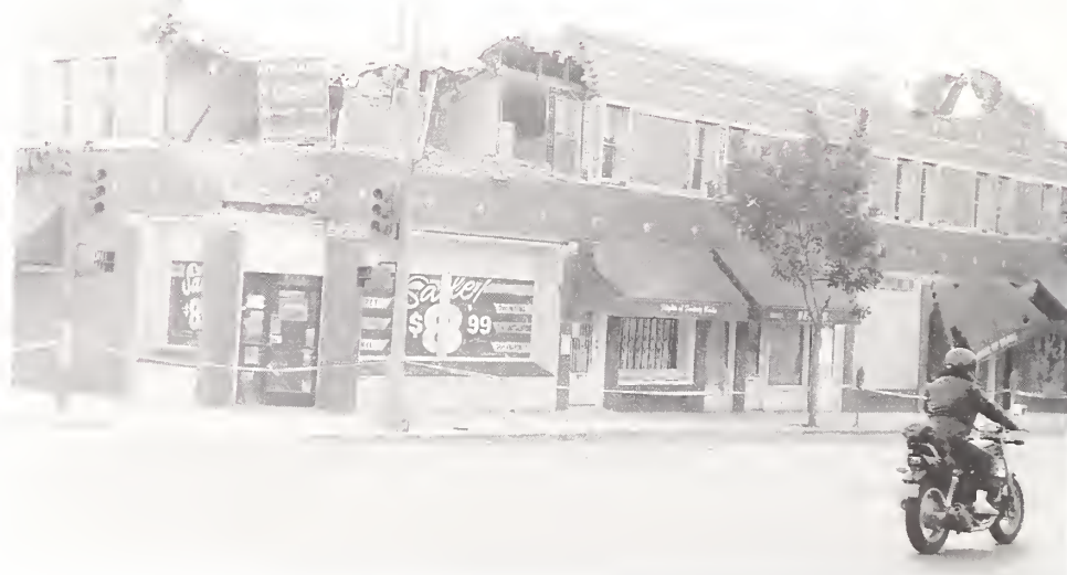
Figure 3.36. Damage to unreinforced masonry buildings, even those that had been rehabilitated, was common. Upper stories and corners were particularly vulnerable to damage. The rows of light-colored diamonds on the face of this building are the end plates of through-bolts used to connect the wall to the floor joists, a typical rehabilitation technique. The remains of parapet braces can be seen on the roof.
