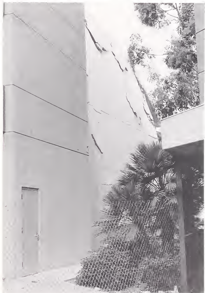
Figure 3.63. At the east and west faces of the Kaiser Permanente Hospital parking garage, shear walls made up the lateral force resisting system. Both walls had horizontal cracks caused by the out-of-plane bending when the walls were pulled inward. Neither wall had major diagonal cracking, suggesting that the lateral load was never fully delivered to the walls. The stair towers remained erect. The east wall and stair tower are shown here.
