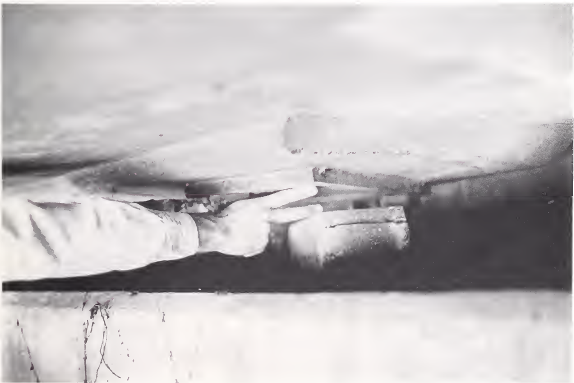
Figure 4.50. Bearing block tipped over at this location resulting in loss of support to girder.
