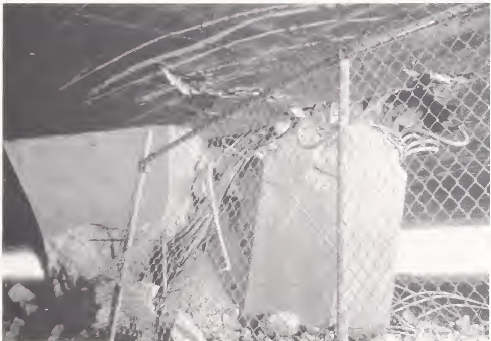
Figure 4.22. Damage to a pier of the SR118 Mission-gothic Undercrossing, looking to the west at Bent 4 of the eastbound bridge, which collapsed (Photo courtesy of EERC).
