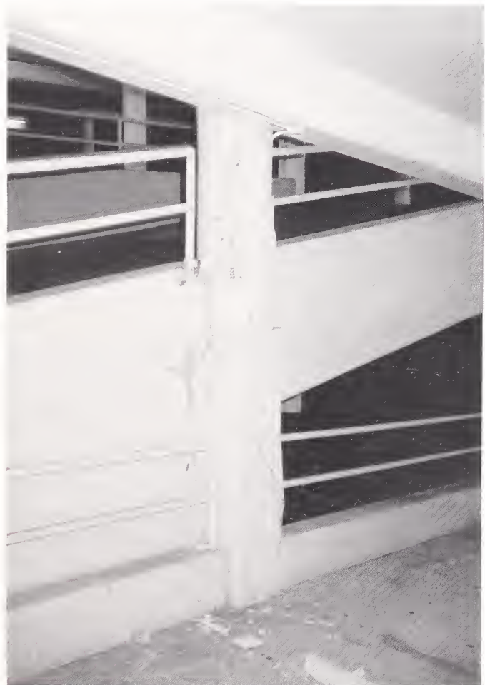
Figure 3.67. In parking garages, ramps can cause unintentionally shortened columns, which are vulnerable to damage, as shown here.
