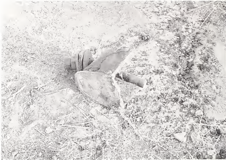
Figure 5.5. Welds of the restrainer brackets broke as the result of strong shaking.
