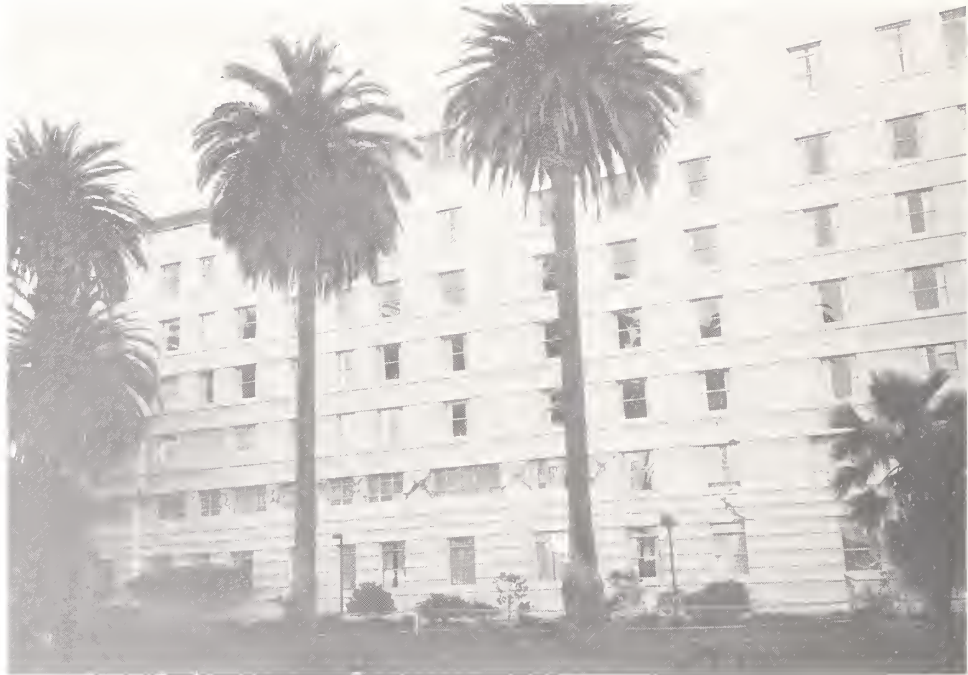
Figure 3.23. The seven-story northwest wing of St. John's hospital in Santa Monica experienced severe X-cracking in the piers between the second story windows.
