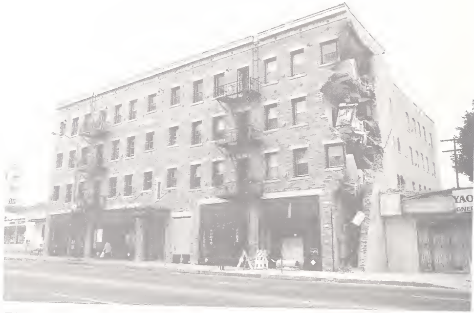
Figure 3.37. The corner of this rehabilitated unreinforced masonry apartment building in East Hollywood crumbled on all four stories.
