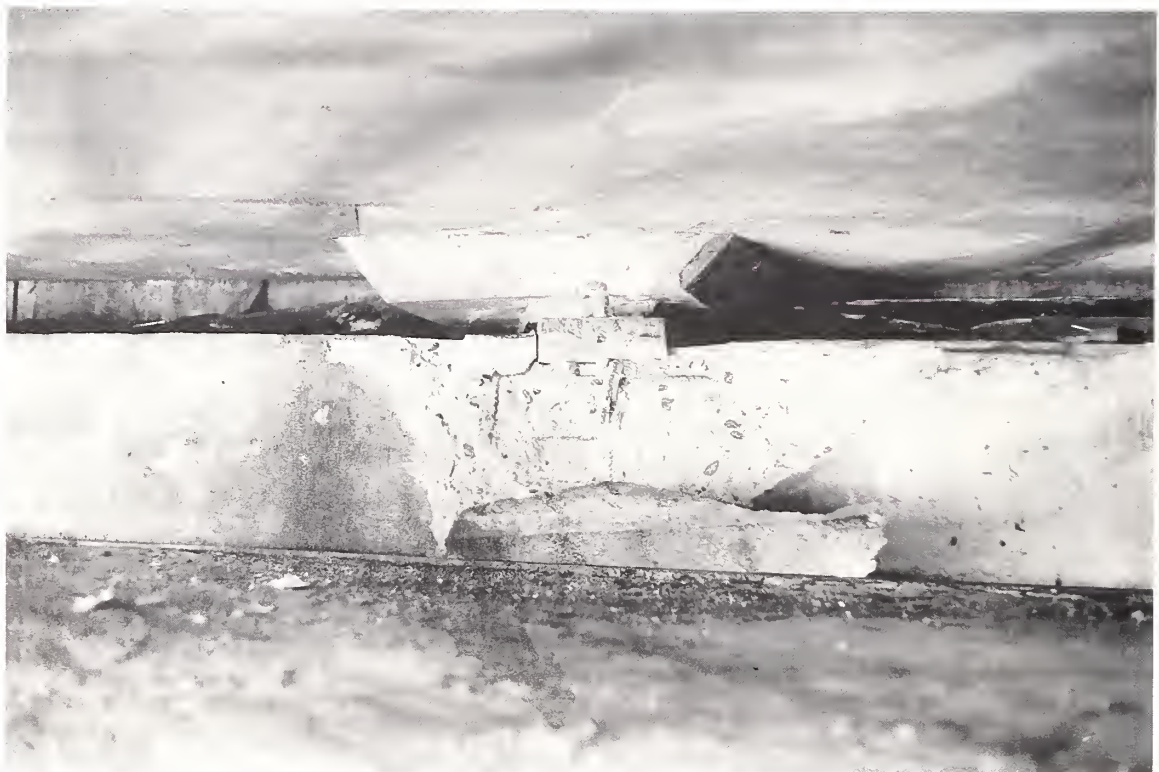
Figure 4.48. Abutment damage at sliding-type bearing.
