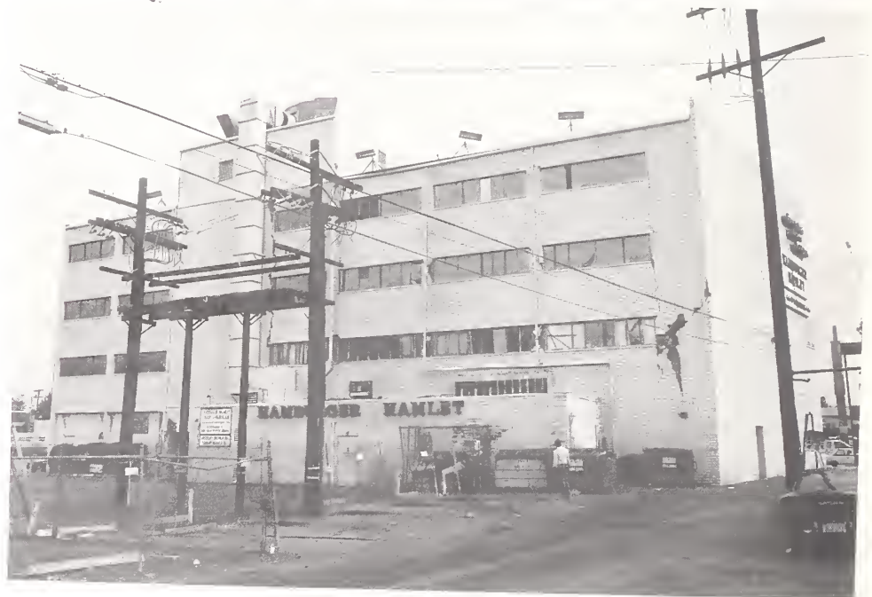
Figure 3.58. The reinforced masonry facade of this steel-framed building in Sherman Oaks was badly damaged.
