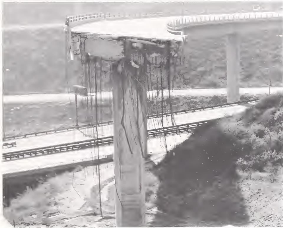
Figure 4.15. View of the flexural failure at Pier 3 of the SR14/I5 North Connector Overcrossing, looking to the south.
