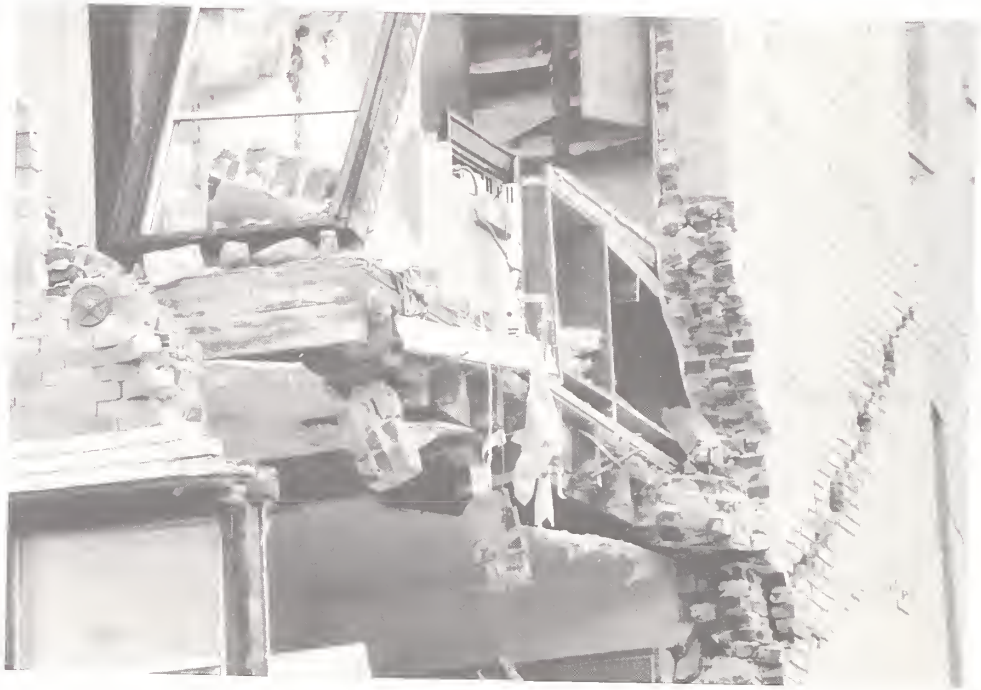
Figure 3.38. A close-up view of the third-story floor diaphragm of the building picture above shows (lower right) a rehabilitation bolt still holding a few bricks to the floor joists, after all the walls on three out of four sides of the bolts had disintegrated.
