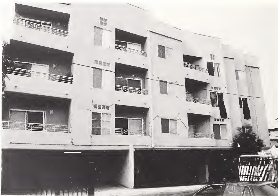
Figure 3.9. Typical damage in to low-rise apartment buildings included diagonal cracks in the stucco facade at the corners of windows and other openings.
