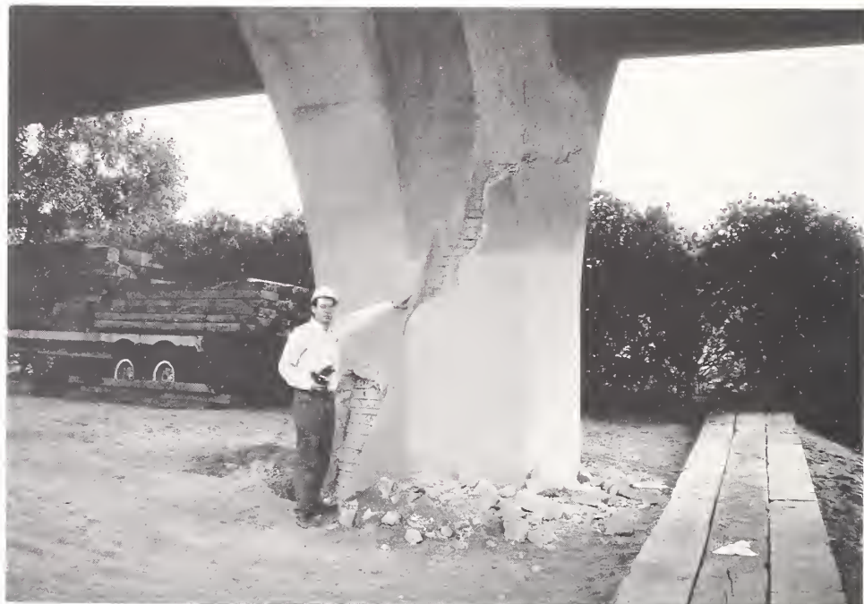
Figure 4.51. View of the westernmost pier at the Interstate 5, State Route 118, Southwest Connector, looking to the southeast. Loose cover concrete has been removed by Caltrans.
