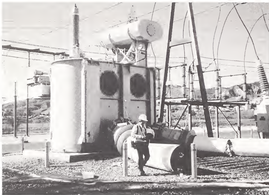
Figure 5.15. Damage to DC equipment at several high voltage substations, such as this one at Sylmar, led to widespread power outages in the Los Angeles area as well as isolated outages throughout seven western states. (Photo courtesy of Edward Matsuda, Pacific Gas and Electric Company.)
