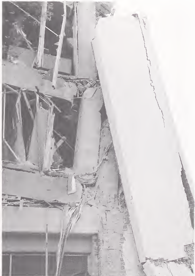
Figure 3.44. The exposed concrete frame of the Kaiser Permanente building, revealing deep beams, suggests that the building had a strong-beam, weak-column configuration. Except for the second story columns, the columns and beams remained intact while the joints disintegrated.
