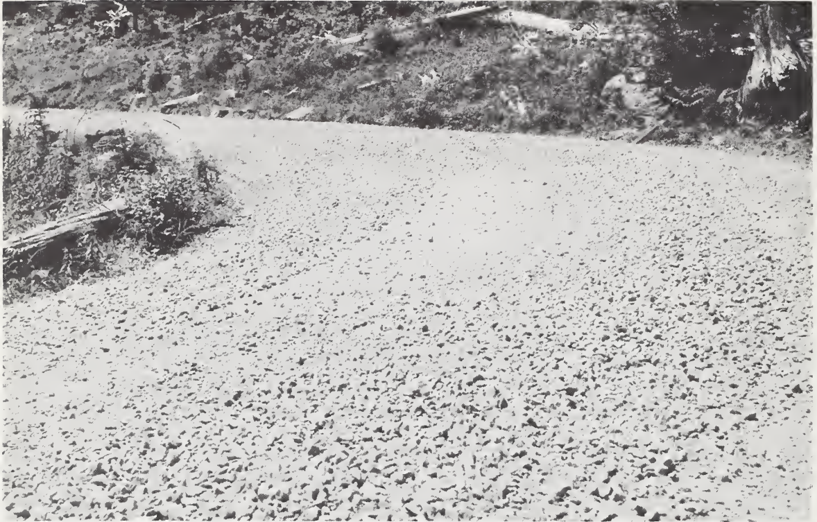
Photo 14.--Permanent forest roads should be surfaced with rock and graded with a center crown to provide for surface drainage. FS Mount Hood photo. No. 6
