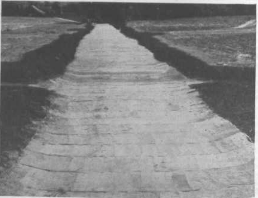
FIGURE 16.—The burlap sacks will give protection in this newly prepared and seeded outlet channel until the vegetation becomes well enough established to carry the run-off safely.
