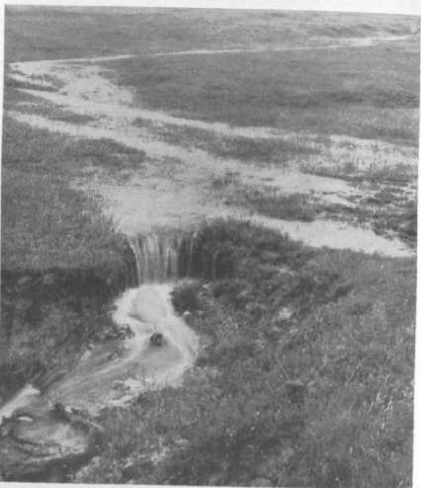
FIGURE 26.—Overgrazing, rodents, mechanical damage, or inadequate maintenance may start overfalls of this type. Unless checked, this overfall will gradually advance and enlarge until the entire drainageway is destroyed.
