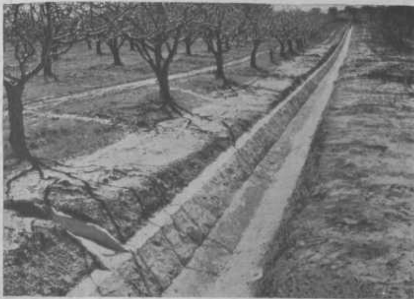
FIGURE 7.—This outlet channel is protected by a continuous lining of rubble masonry.
