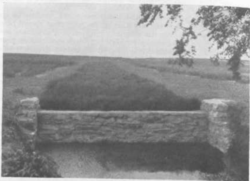
FIGURE 24.—A masonry structure has been used at the lower end of the channel to carry the run-off over a critical overfall to a stabilized drainageway.
