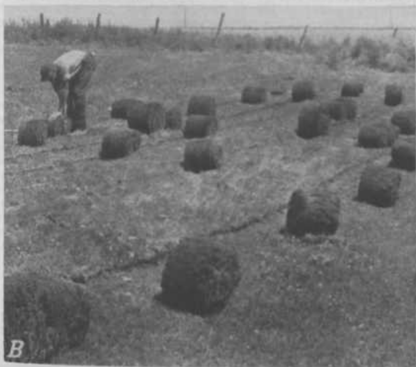
FIGURE 20.—A, Sod is being transplanted over this outlet channel in order to get a protective covering immediately; B, the sod has been cut and rolled preparatory to transportation to an area that is to be sodded.
