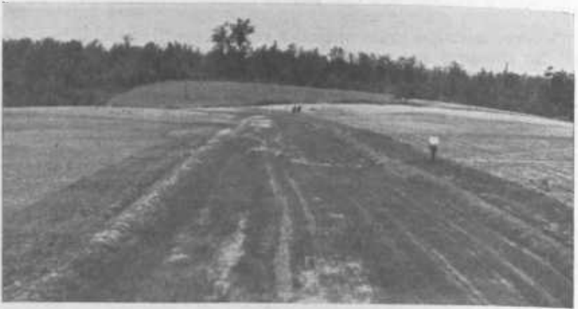
FIGURE 17.—This drainageway has been shaped to proper cross section and seeded for run-off disposal. Note the small earth embankments along the sides, used to protect temporarily the seedbed and young plants.
