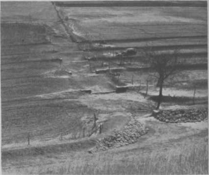
FIGURE 6.—Drop-check structures reduce the grade of this terrace-outlet channel. The run-off is slowed down.
