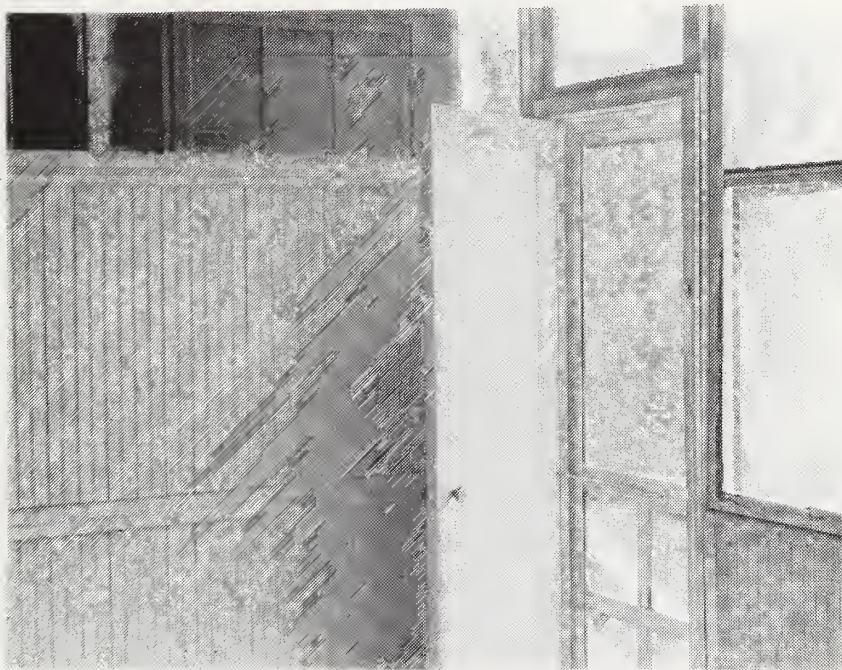
Figure 17. Interior view of wall and door of screened porch after removal of old paint and repainting.
