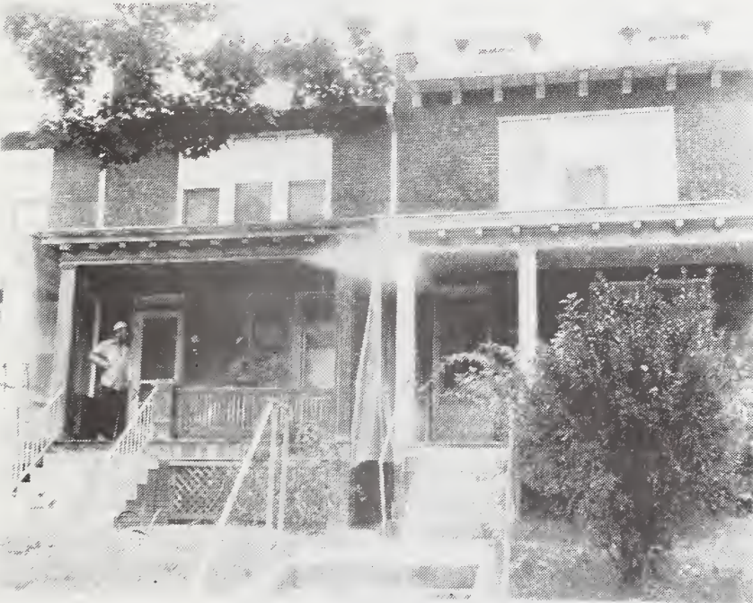
Figure 10. Flushing off old paint with high pressure water spray after treatment with paint remover. Note water overspray onto adjoining porch.
