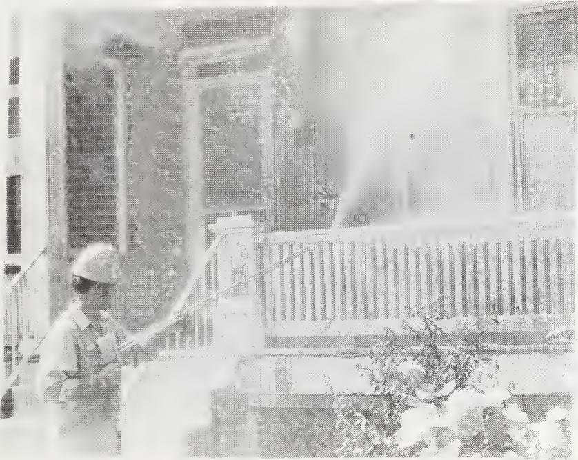
Figure 9. Flushing off old paint with high pressure water spray after treatment with paint remover.
