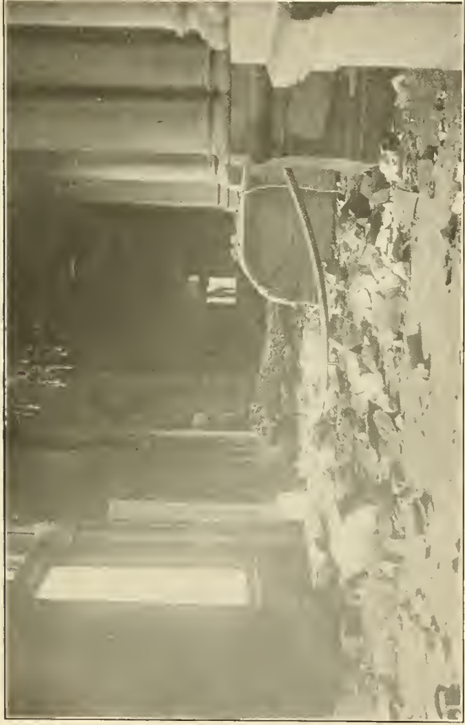
Fourth floor, corridor on northern side of Great Western Staircase, showing stones that have fallen from the side ceiling, owing to the intense heat
