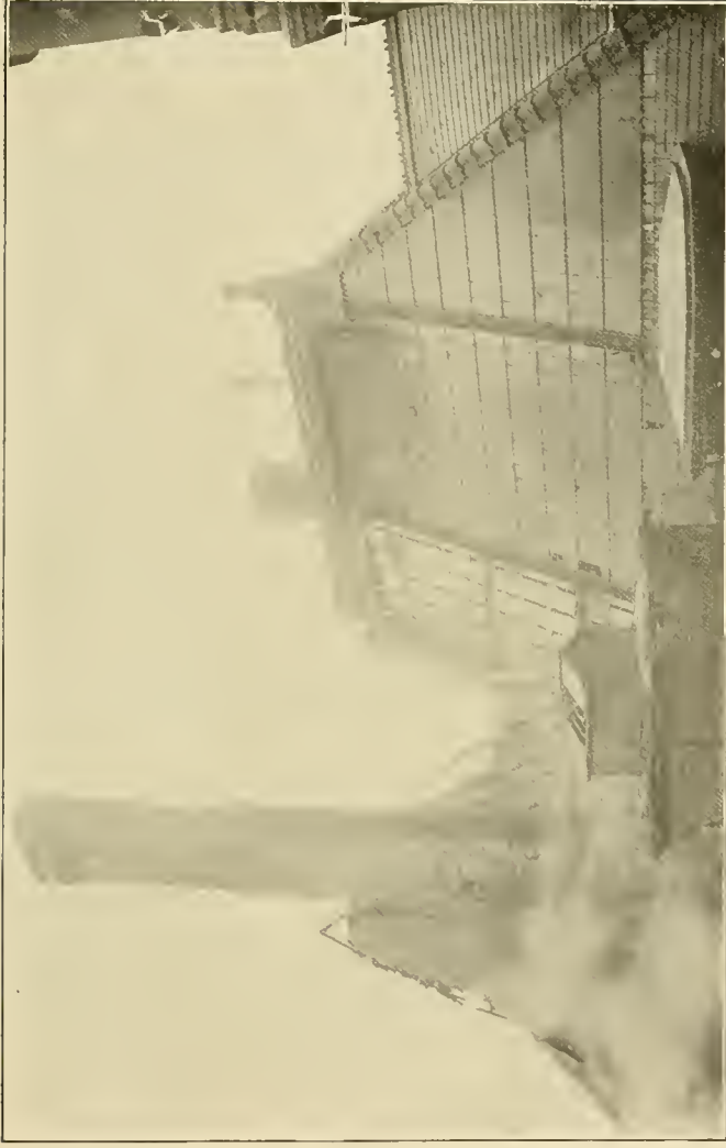
Roof of the Great Western Staircase looking south from the Washington Avenue side of Capitol The State Street half of the roof had fallen
