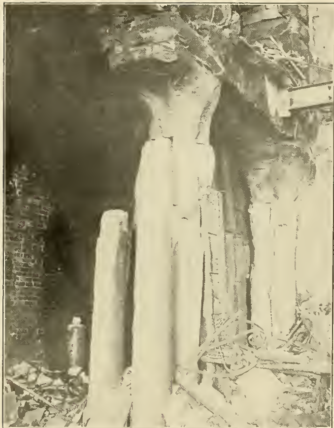
Near view of the red granite columns in the northeastern corner of the reading room of State Library, entirely destroyed by the heat
