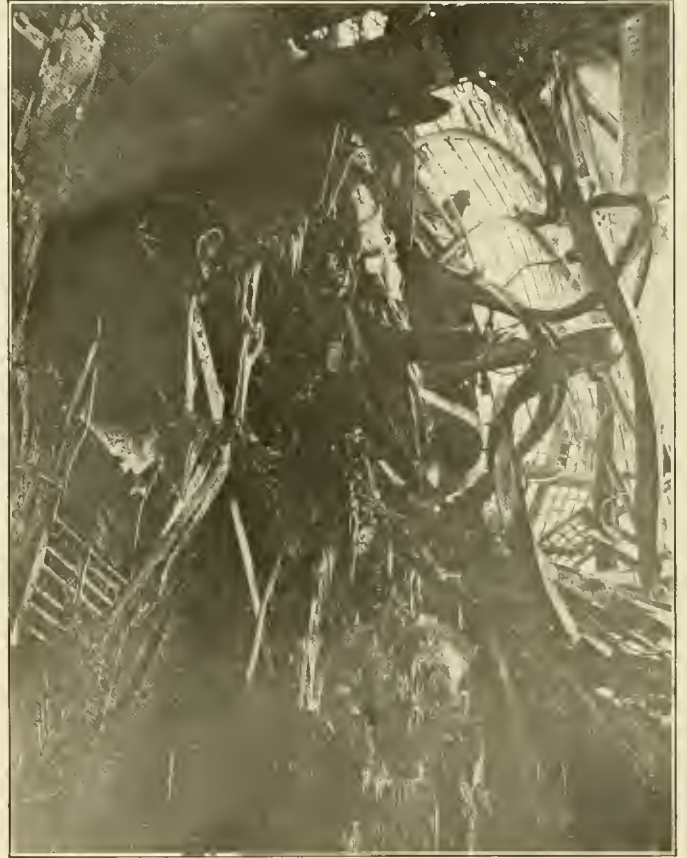
The effect fire had on the iron work
