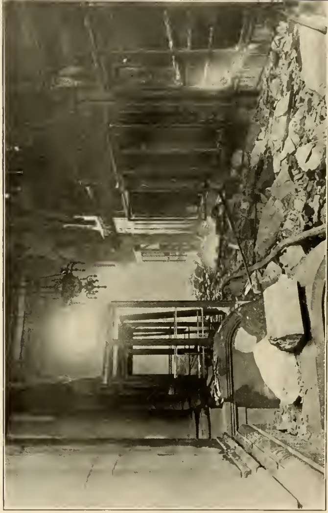
Fourth floor, corridor on Southwest Staircase; the cases contained valuable Indian Curios. The intense heat caused the stones to fall from sides and ceiling; the electric-light bulbs in the chandeliers were not broken
