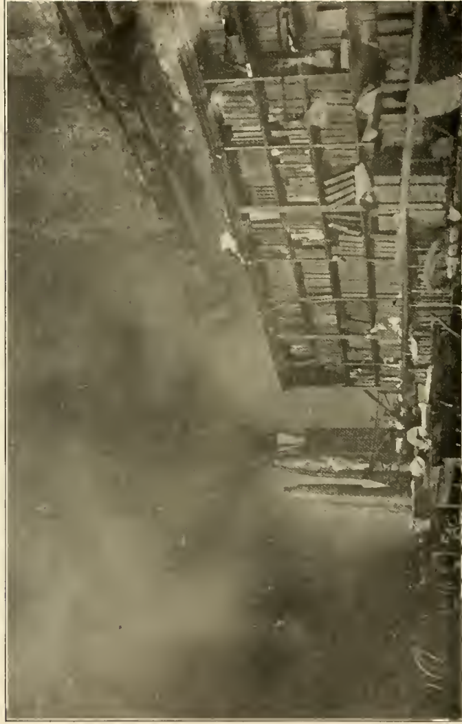
Main reading room, State Library, looking toward northeast corner, showing steel beams of mezzanine floor, also beautiful red granite columns entirely ruined by the fire
