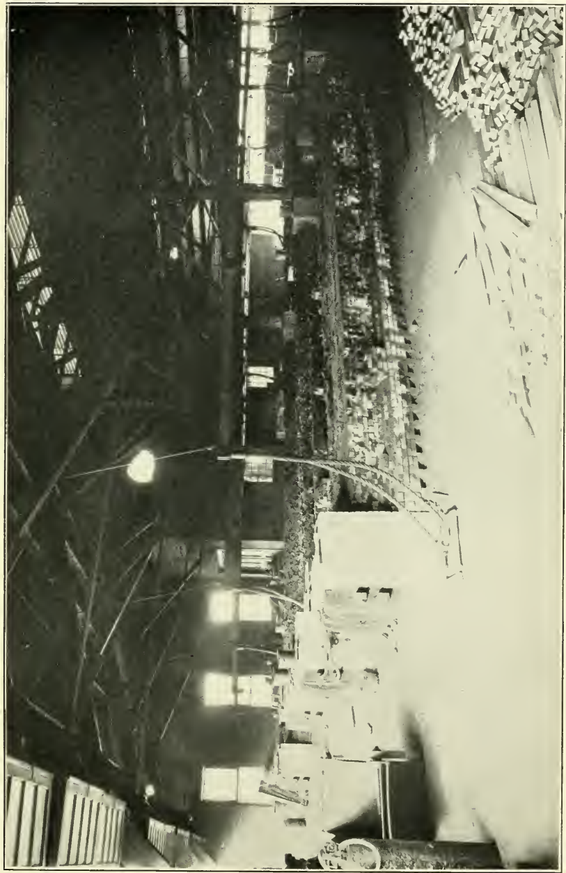
INTERIOR OF FURNACE ROOM, INTERNATIONAL ACHESON GRAPHITE COMPANY, NIAGARA FALLS, N. Y.
