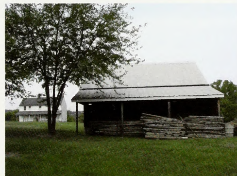
NPS recently restored historic buildings damaged during a storm at the Lewis Farm on Monocacy National Battlefield in Maryland.
