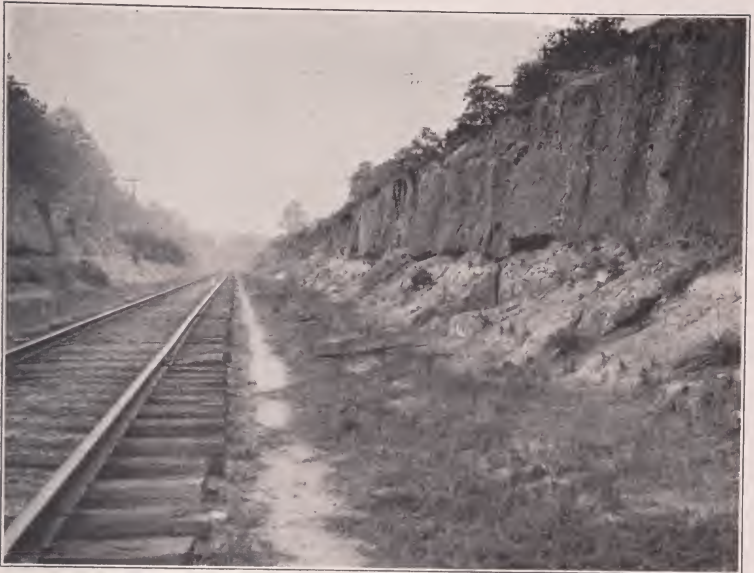
A. CUT OF ATLANTIC COAST LINE RAILROAD WEST OF CLIMAX, DECATUR COUNTY, SHOWING STRATA OF THE ALTAMAHA FORMATION.
