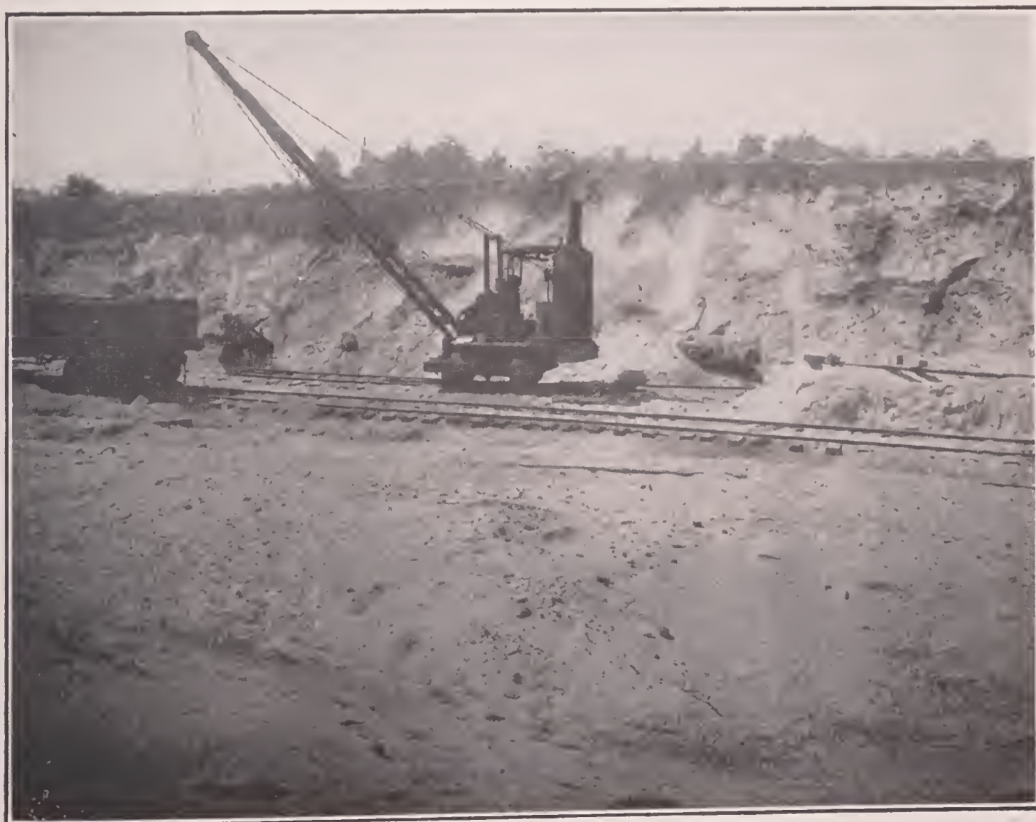
B. EXPOSURE OF RESIDUAL, SURFICIAL SAND IN A SAND PIT NEAR HOWARD, TAYLOR COUNTY.
