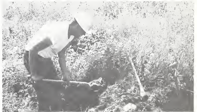
Steve Howlett, member of the Flathead Tribe, at work on excavation for irrigation structure (Courtesy, Bureau of Indian Affairs—Department of the Interior).
