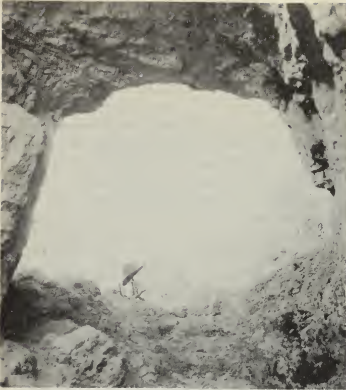
Photograph 19. -Caves, arches and tunnels in the clay banks of draws are common in the Bighorn Basin. This one is on Wildhorse Draw. They are caused by water acting on unstable soils.
