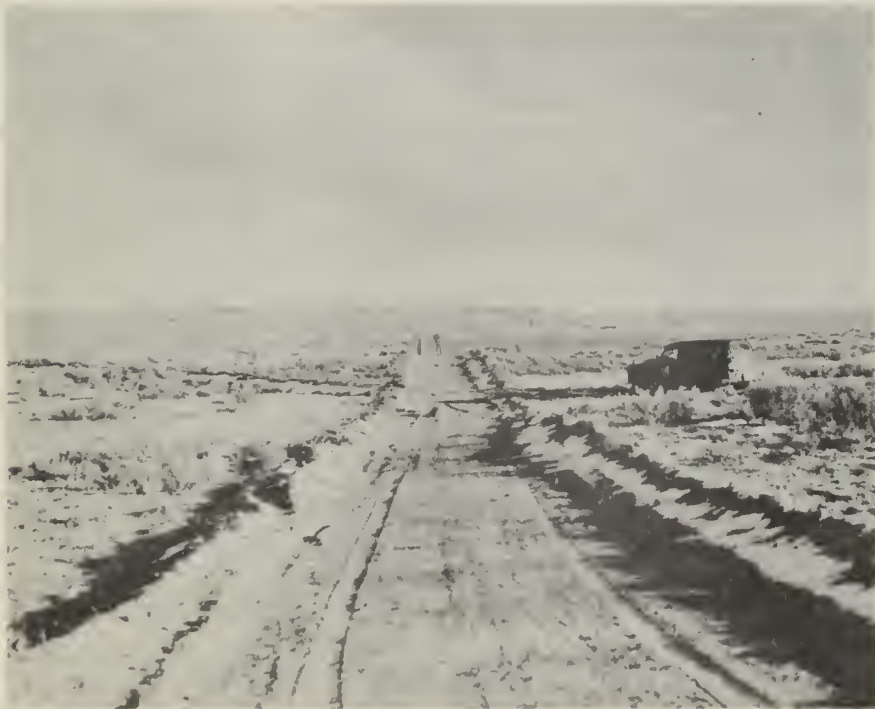
Photograph 15. -Seismograph "roads" built with a bulldozer averaging from six to eighteen inches deep. In this area it would have been necessary only to remove the sagebrush.
