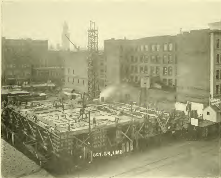
THE BUILDING IN PROCESS OF CONSTRUCTION, SHOWING METHOD EMPLOYED BY CONCRETE ENGINEERING CO.
