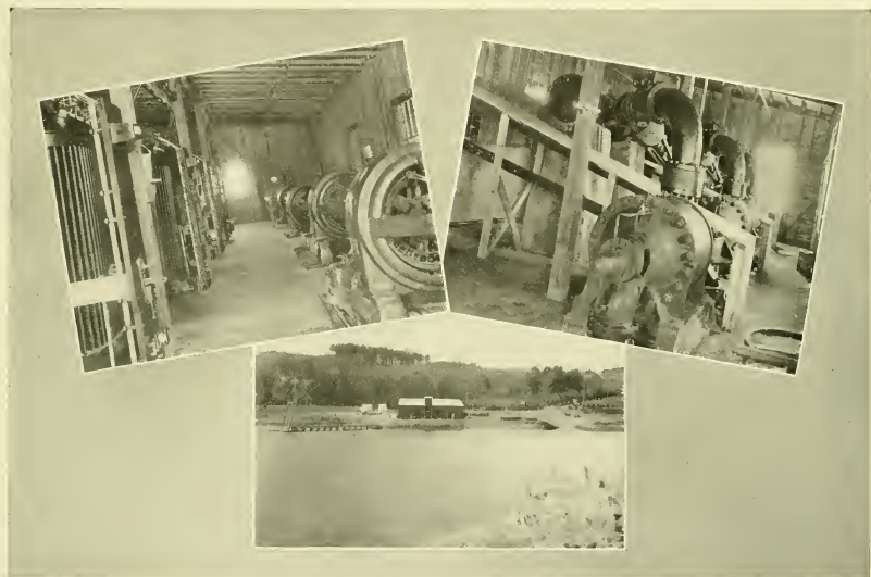
THE EMERGENCY PUMPING PLANT AT THE METROPOLITAN BASIN
