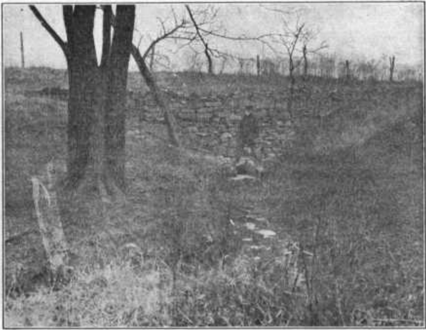
FIG. 25.—Lower side of soil-saving dam, showing end of outlet pipe discharging into a concrete trough to prevent washing below the dam.
