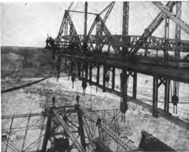
ERECTING GANG AT WORK ON THE TRAVELING CRANE AT THE LETHBRIDGE VIADUCT, SOUTHERN ALBERTA.
