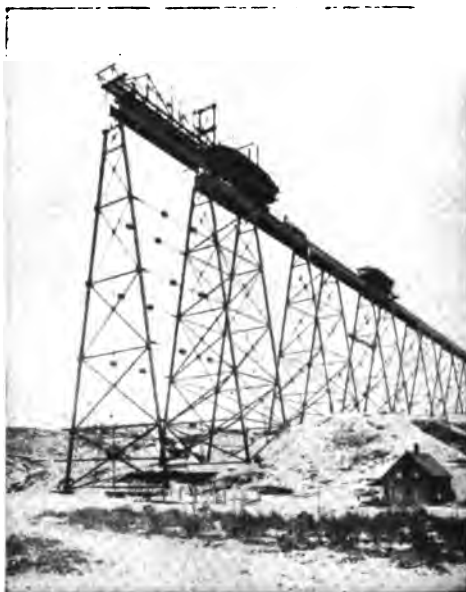
THE LETHBRIDGE VIADUCT WHICH IS MARCHING ACROSS THE VALLEY OF THE BOW RIVER. It will be a mile-long and 320 feet high.
