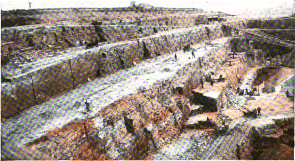
A STONE QUARRY. FROM WHICH THE MATERIAL IS CUT IN SUCH A WAY THAT TERRACES ARE FORMED. RENDERING THE WORK LESS HAZARDOUS. The stone is then removed by means of inclined planes and electric hoists.
