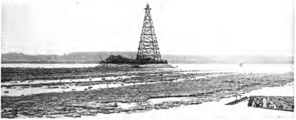
A PORTION OF THE COFFERDAM, SHOWING, IN THE LEFT FORE-GROUND, THE BED OF THE DETROIT RIVER EXPOSED.
