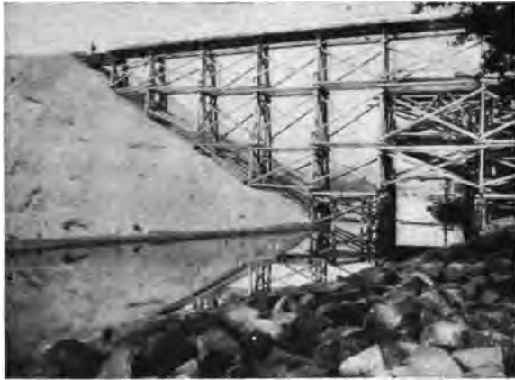
BUILDING THE SAND DAM ACROSS THE STOESENSEE. The trestle bears trains transporting sand.
