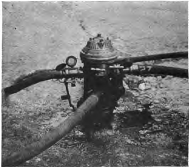
HYDRANT WITH HIGH PRESSURE GAUGES. Control of the water's force is easy with these recording instruments as aids.
