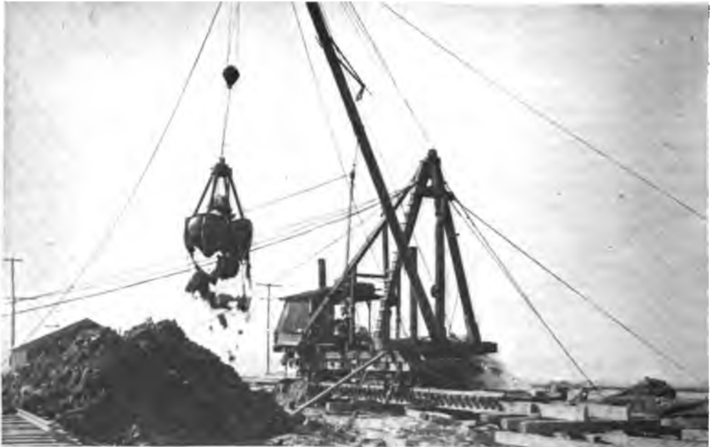
EXCAVATING QUICKSAND INSIDE OF COFFERDAM FOR THE PIERS OF A DRAWBRIDGE IN A LOST CHANNEL.
