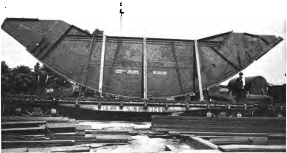
JUST A PART OF THE HARD-LUCK BRIDGE. THE ROCKER ON WHICH THE LONG DRAW ROLLS.
