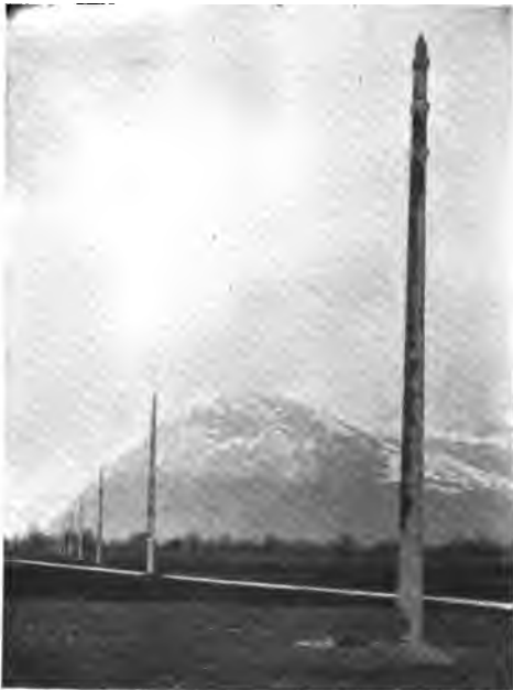
CONCRETE POLES IN USE IN CONNECTION WITH THE ALBULA POWER TRANSMISSION PLANT, SWITZERLAND.
