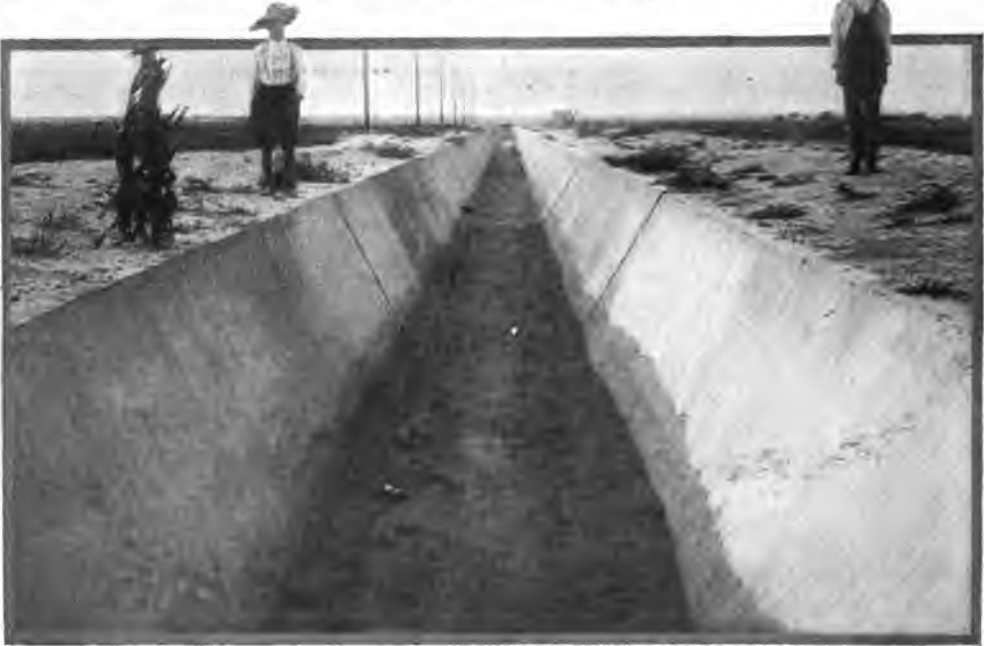
THE MAIN CANAL AS IT APPEARED COMPLETED AND STILL FREE FROM WATER.
