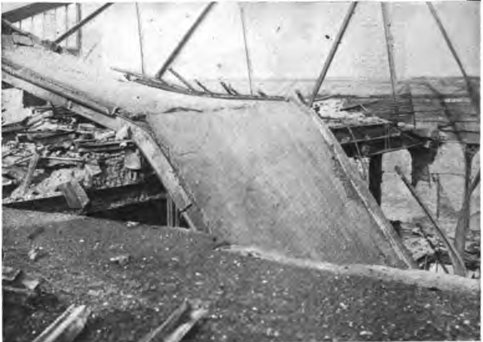
A COLLAPSE IN THE PARKER BUILDING, CAUSED BY FAILURE OF UNPROTECTED STEEL COLUMN TO WITHSTAND THE HEAT.
