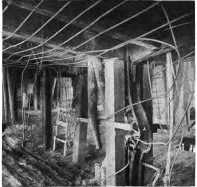
A DISTORTED STEEL COLUMN, "A." THE RESULT OF WARPING FROM INSUFFICIENT FIRE PROTECTION.
