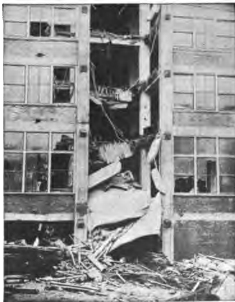
PART OF WRECKAGE MADE BY FALLING TANK, SHOWING DAMAGE DONE TO CONCRETE FLOORS.
