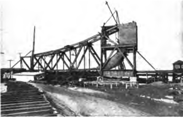
A VIEW SHOWING THE DRY LAND OVER WHICH A RAILROAD WAS COMPELLED BY THE GOVERNMENT TO THROW A $200,000 DRAWBRIDGE.
