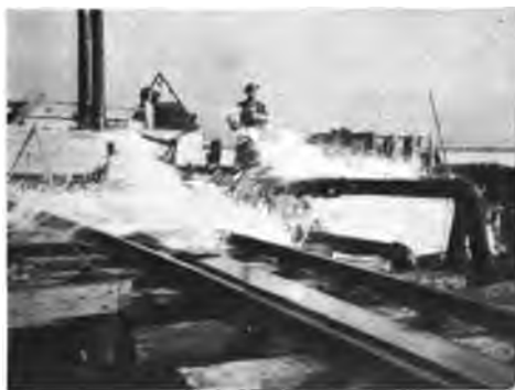
THROUGH THIS AIR LIFT 2,000,000 GALLONS OF WATER PASSED EVERY HOUR.
