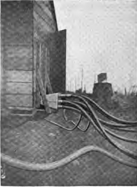
THE TWELVE SECTIONS OF RUBBER HOSE THROUGH WHICH AIR FANS THE BLAZE AT THE BASE OF THE STUMPS.
