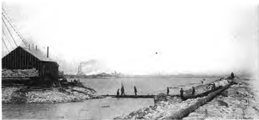
ANOTHER PART OF THE WORKS. SHOWING PIPING THROUGH WHICH A CONSIDERABLE AREA WAS PUMPED DRY.
