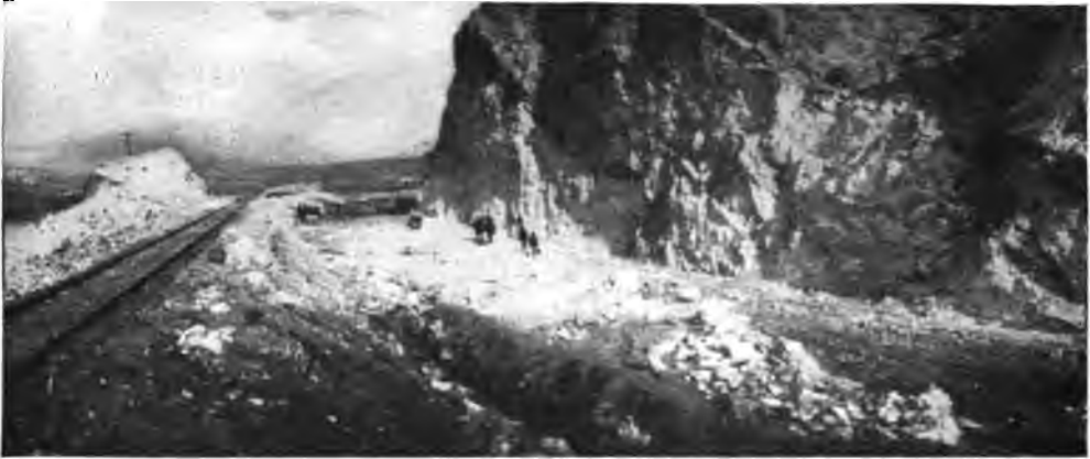
CUTTING THE END OFF A MOUNTAIN RANGE AND DIGGING A CANAL THROUGH STONE. TO CARRY THE WATERS OF THE MEADOW VALLEY RIVER BETWEEN THE ROADBED AND THE MOUNTAIN WALL.
