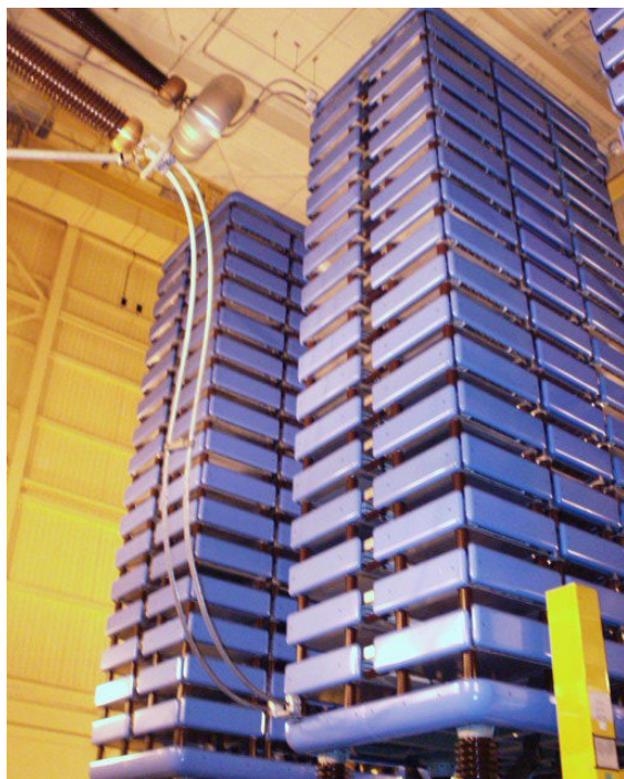
Valve hall containing thyristor valve stacks used for long distance transmission of power from Manitoba Hydro dams
