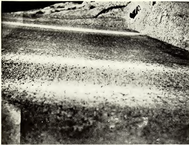
UP ON THE LEDGE (The white bands in the photograph show how the inscription has been damaged by the water)
