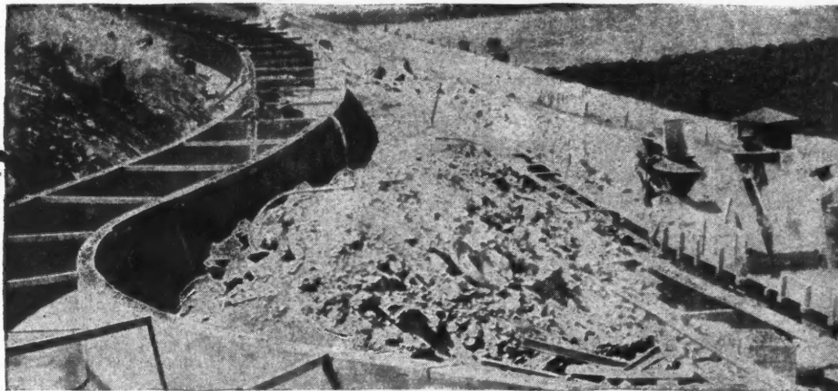
Lindsay-Strathmore irrigation district, San Joaquin Valley, Cal.—2-in. "Gunite" walls, reinforced with wire mesh.
