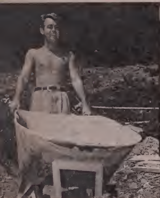
Alan finds hauling cement a wonderful way to keep fit and get a house built.
