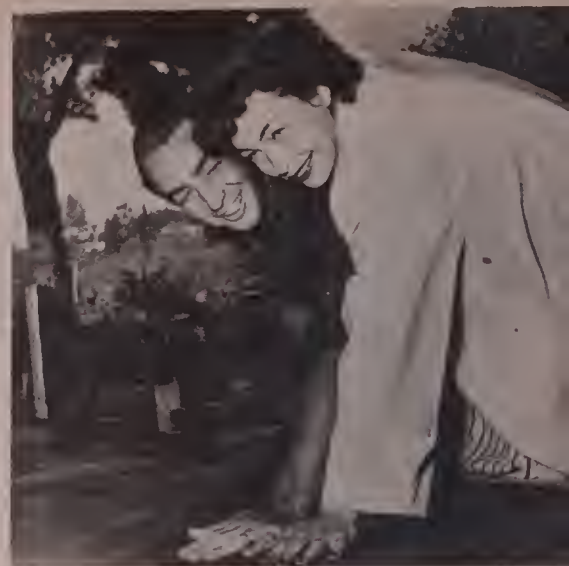
Patio gets a final layer of cement; also a set of handprints: Betty's and Mac's.
