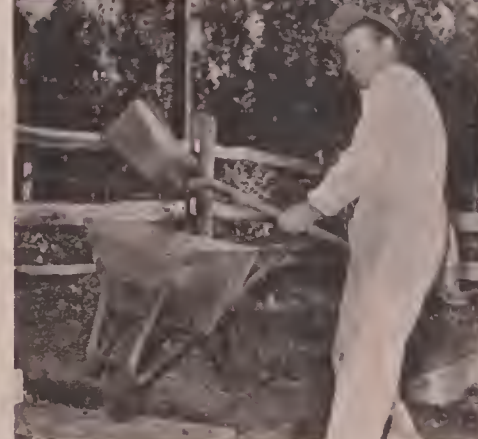
When Don takes to his saw and hammer, a fence is up in no time. Next project, a garden. It makes me tired just to watch.
