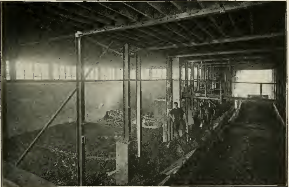
Clay storage and receiving room. Toronto-Hamilton Sewer Pipe Co., Ltd.
