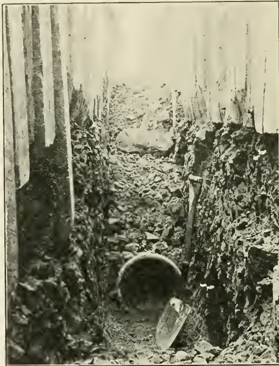
Sewer trench, showing careless back filling over freshly-laid sewer.
