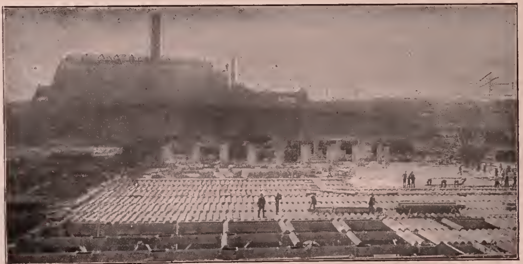
Fig. 47—View Illustrating Form Construction for Bush Terminal Factory. See Fig. 42 for Finish View.
