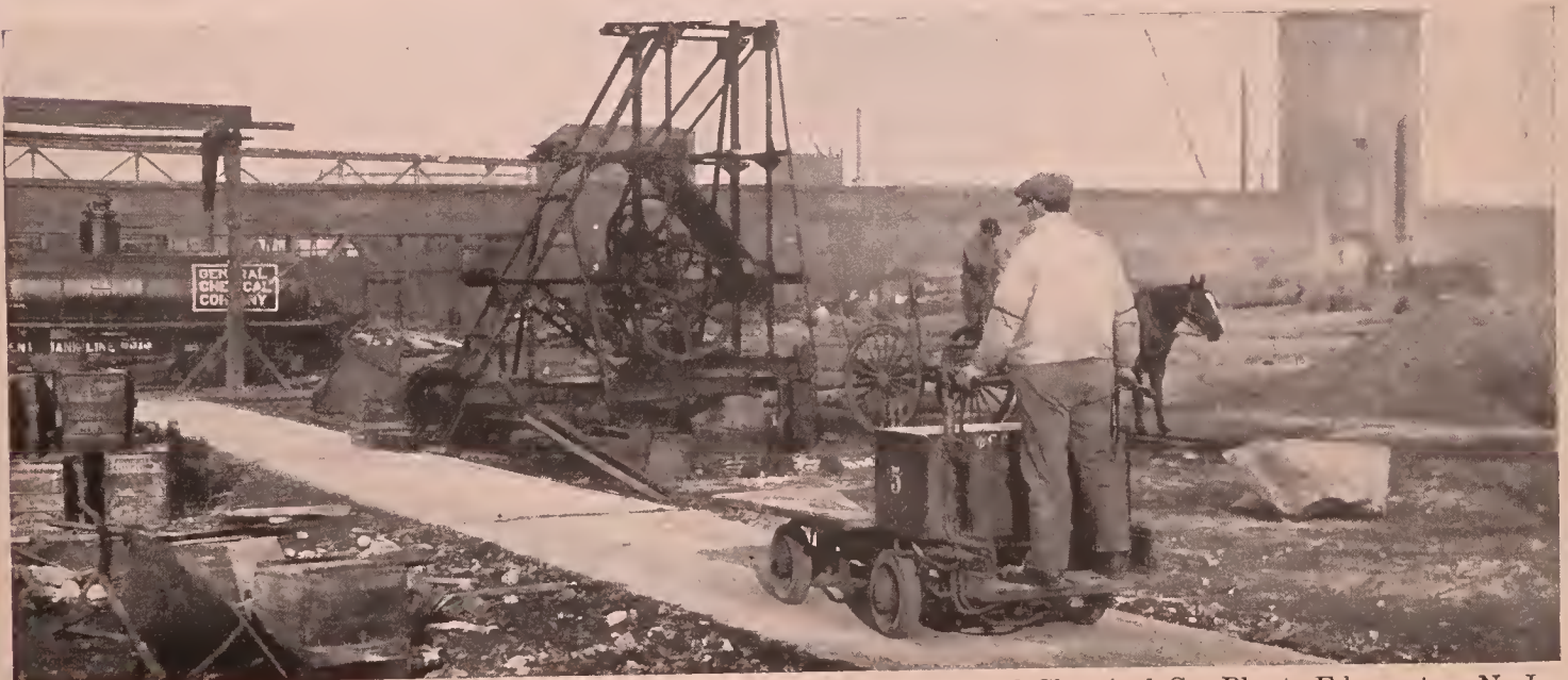
Part of the System of Concrete Driveways and Walks at the General Chemical Co. Plant, Edgewater, N. J.
