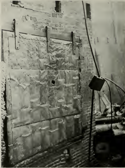
A Standard Fire Door. —In a large paper warehouse in which everything in one section was destroyed by fire, a line of standard tin-clad fire doors effectively protected all stories of the adjoining section. The accompanying photograph shows one of the doors. Self-releasing timbers saved the walls from wreck, and the doors kept the fire in the burning section. Note the integrity of the standard hardware and the unwarped body of the door due to its well selected lumber and proper nailing. Nothing happened to it but the bite the fire took out of the core exposed in the little round gas-vent.
