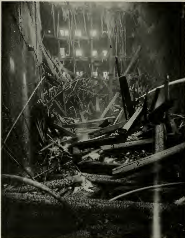
Dry Rot in Timbers. —Shortly after the fire was under control the floors began to fall in irregular sections, and in two or three hours the whole floor system of the large building had fallen in a tangled mass to the basement. The reason of this collapse is indicated by the condition shown in timbers numbered 1 to 6.
