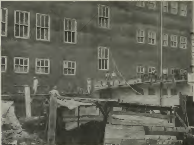
ANOTHER PICTURE OF WATERPROOFING PROCESS UNDER WAY AT THE HALE DEPARTMENT STORE, SAN FRANCISCO Reid Bros., Architects
