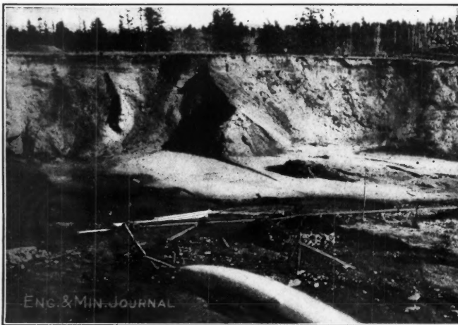
FIG. 3. THE HYDRAULIC STRIPPING PIT FROM THE EDGE OF THE HIGH SLUICED PIT
