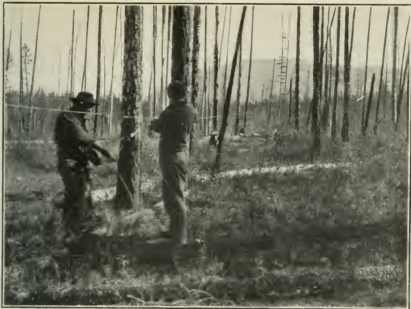
FIG. 1.—SAVING MANY LONG, HARD TRIPS AND TIME BY ESTABLISHING TELEPHONE COMMUNICATION. [Strung to trees by forest officers.]
