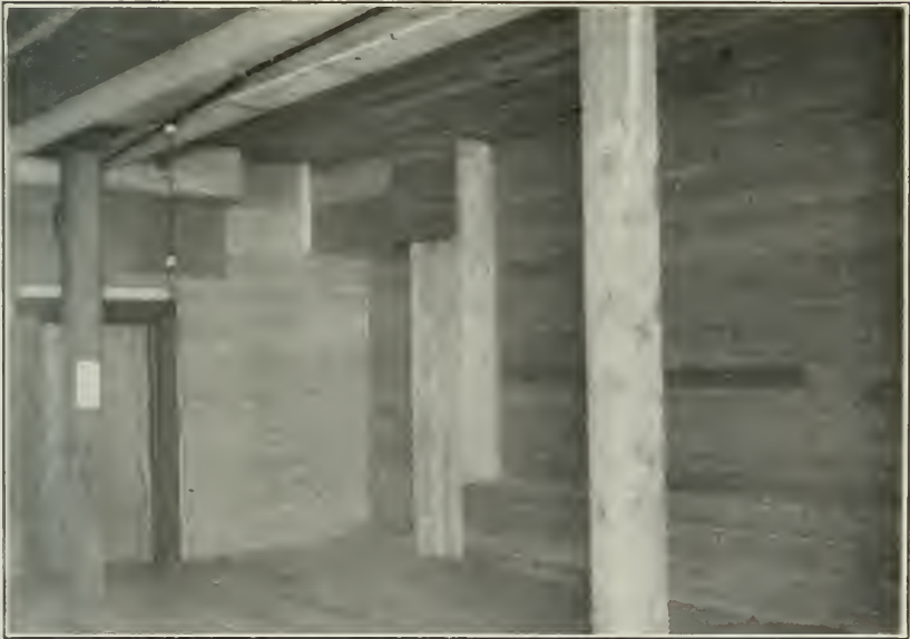
FIG. 2.—PRECOOLING ROOM IN AN ORANGE-PACKING HOUSE AT UPLAND, CAL., SHOWING AIR DUCTS FOR DISTRIBUTING COLD AIR THROUGH PERFORATED FALSE FLOOR AND CEILING.
