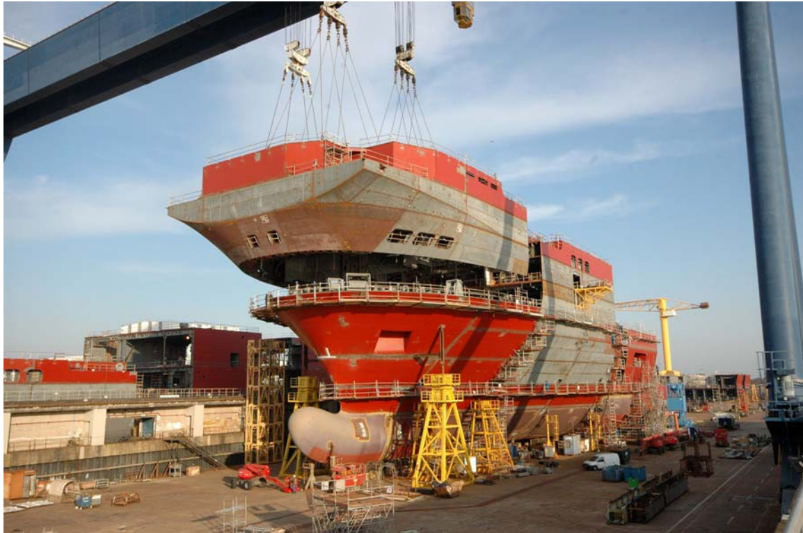
Figure 8. Example of the modular construction of the Mistral BPCs. This is the 690 ton forward module being assembled for the third French BPC, the Dixmude . (From Bernard Biger, STX France, 2009) 76
