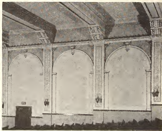
Panels between plaster-ornamented pilasters in the Hiland theatre, Fort Thomas, Ky., treated with U. S. Gypsum acoustic tiles.
