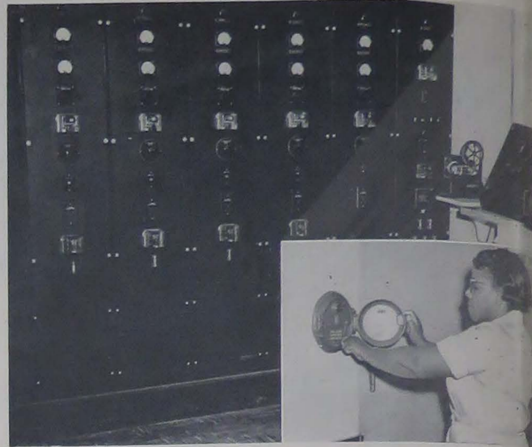
Inset, right, A ward attendant sounds the fire alarm. In case of fire this is the first action to be taken by personnel in the vicinity of the fire. Main picture shows equipment located in the fire department quarters which receives and records fire alarms.
