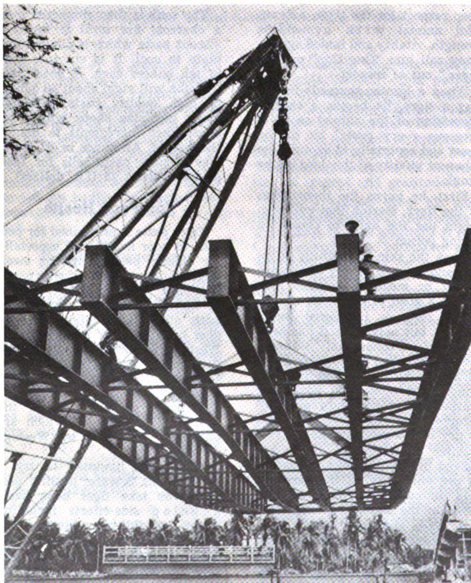
Construction of one of many bridges in South Vietnam by RMK-BRJ firm.
