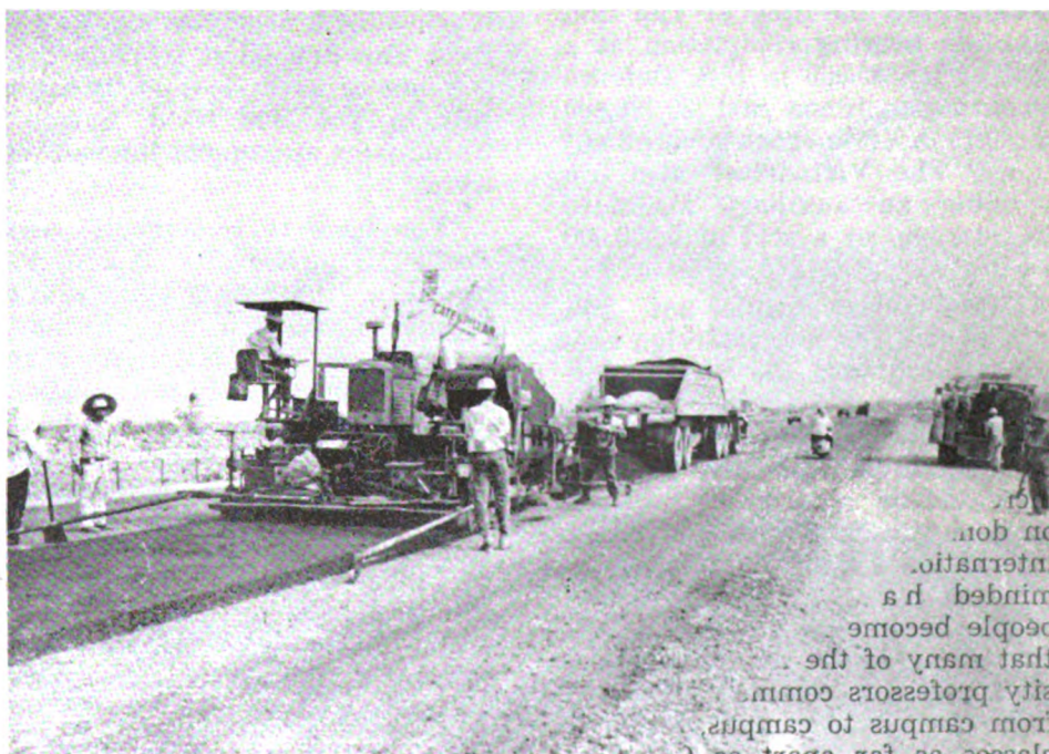
Four thousand kilometers of main highways are being reconstructed throughout Vietnam in a project that has already upgraded some 2,500 kilometers.
