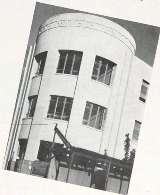
Tower complete except for doorways as the George H. Clark building nears completion during the summer, 1946.
