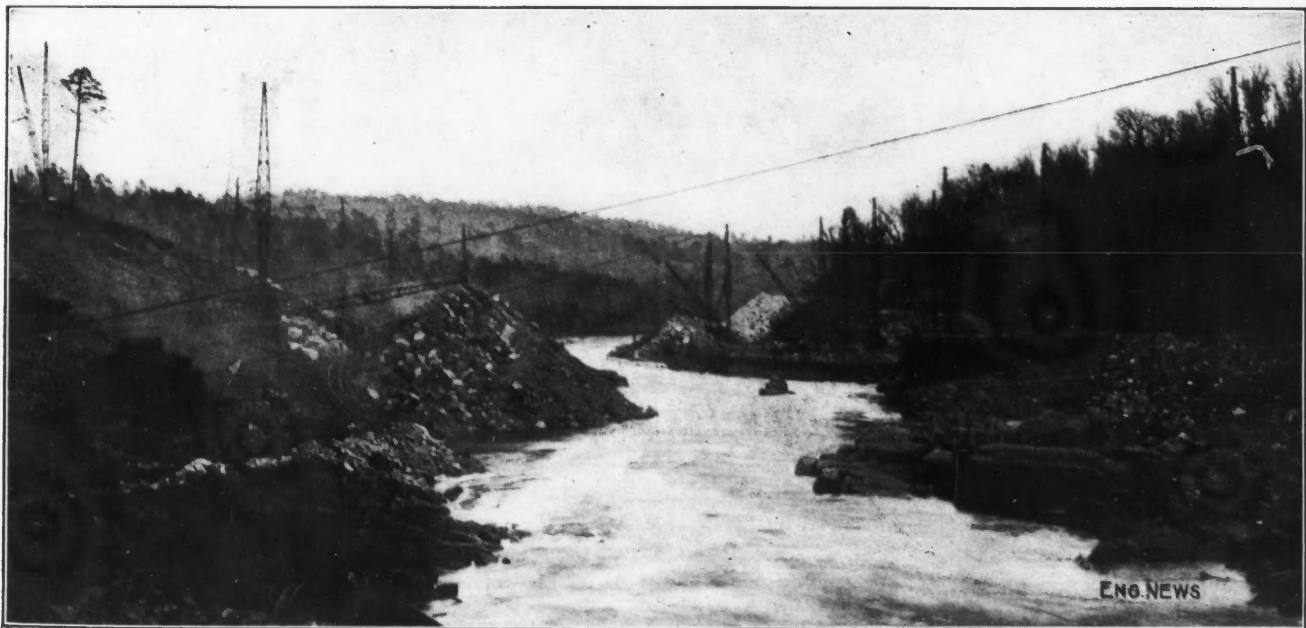
SITE OF SOUTH ALUMINIUM CO.'S NEW DAM, LOOKING DOWNSTREAM Tunnel portal at left, coffer-dam cribbing at right.
