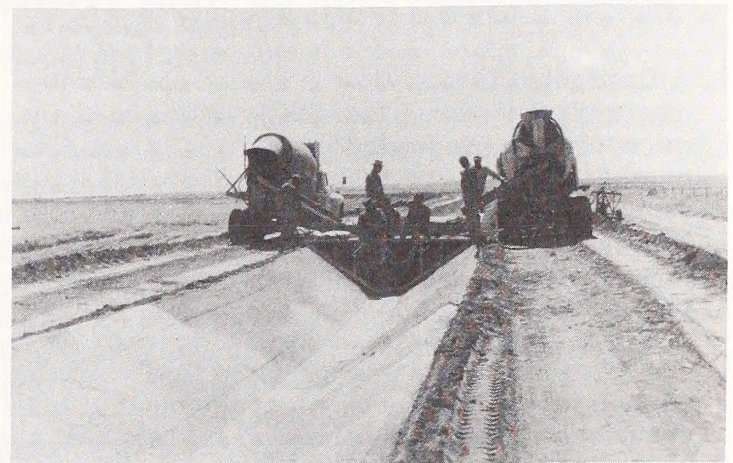
A concrete ditch minimizes water loss from seepage, but is expensive to construct.
