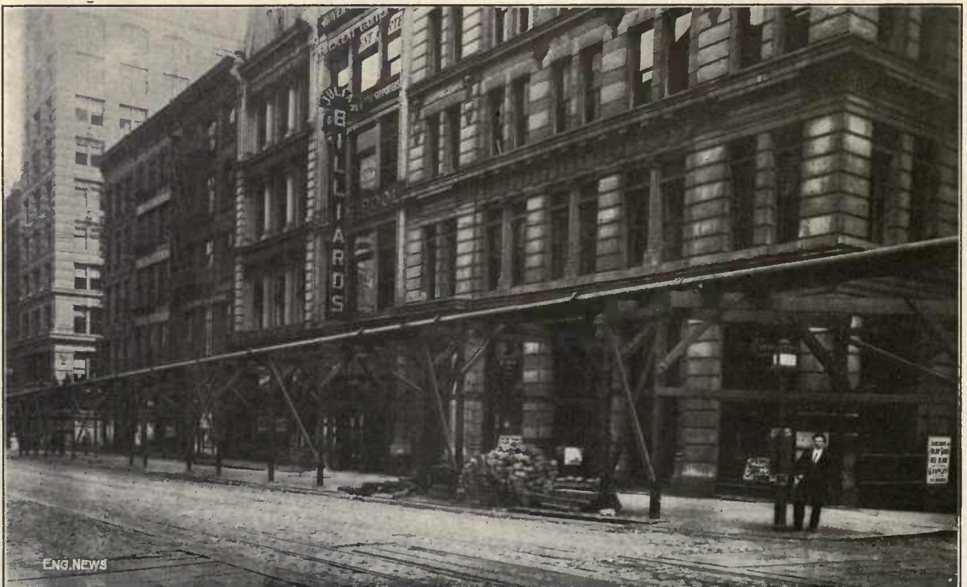
FIG. 28. OVERHEAD GAS MAIN ON LOWER BROADWAY
