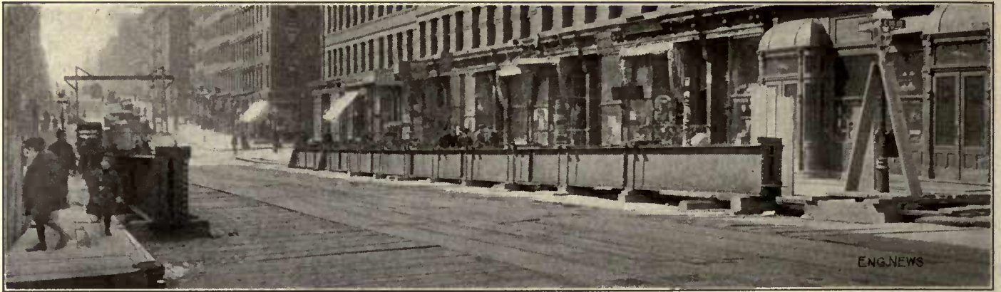
FIG. 36. STEEL GIRDERS ON STREET SURFACE CARRYING TIMBERING AND DECKING, LEXINGTON AVE., SECTION 11, ROUTE 5.
