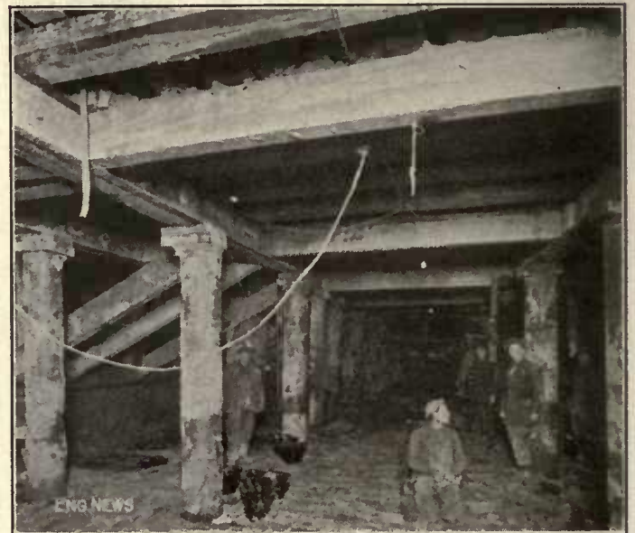
FIG. 37. STREET DECKING AND TIMBERING CARRIED ON HOLLOW STEEL PILES UNDER CHURCH ST., SECTION 1, ROUTE 5
