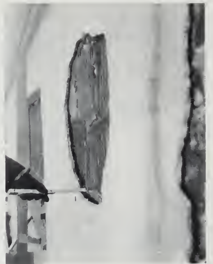
Here everything was wrong. Partition tile instead of that for a stucco base was used and the wrong waterproofing was applied, preventing bonding of the stucco
