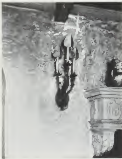
A wall crack that cost several hundred dollars to repair. Under the plaster the studs and lath had rotted badly and the electric wires had become short circuited
