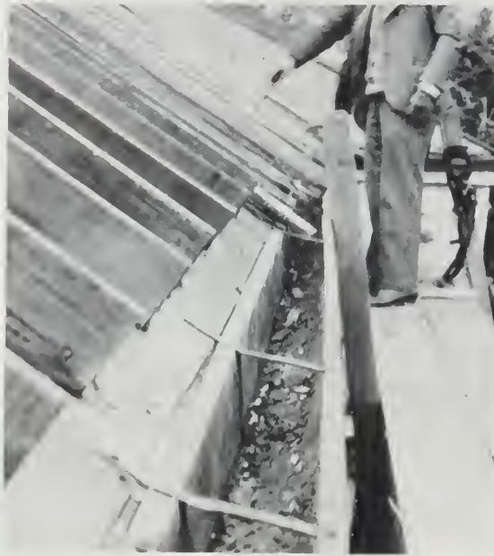
The wrong way to install a gutter. It has too narrow a lap and, as the roofing paper was not brought down to meet the gutter, water blew up under the eaves and found its way into the walls to cause disastrous leaks
