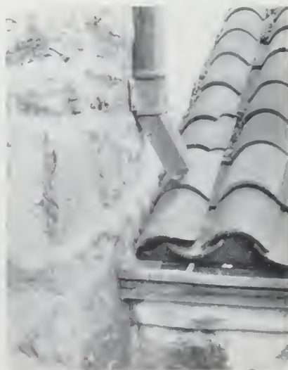
A downspout improperly located. Water, discharged into the intersection between roof and wall where there was no flashing, seeped into the walls, causing a succession of leaks
