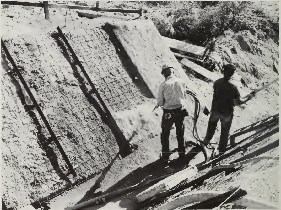
Structures (such as this concrete flume) have been built by SEA employees to measure runoff from watersheds from 1 acre to 58-square miles in size.
