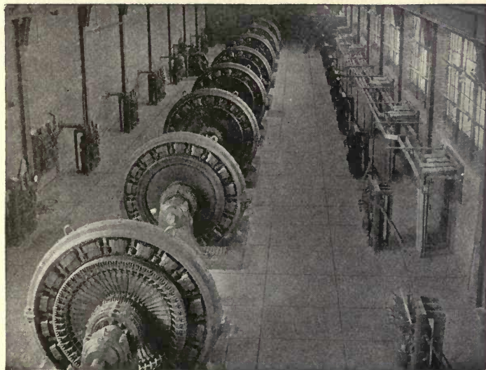
FIG. 51. Nine 2500-kw. converters used to supply current for the production of aluminum. There are thirty-six similar machines installed in the Marysville, Tenn. Plant of the Aluminum Co. of America. Westinghouse Electric and Mfg. Co.
