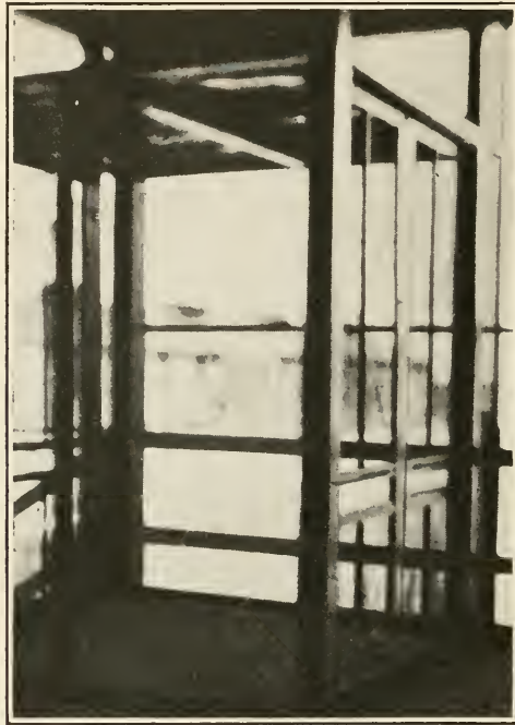
FIG. 140.—Vestibule to porch with double screen doors, shown on right and extreme left, the outer doors being at the left. The screening material does not show up very plainly.
