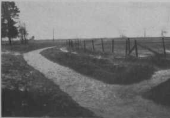
FIGURE 10.—Water from more than 100 terraced acres has been carried safely to a stabilized drainage in sodded outlet channels.
