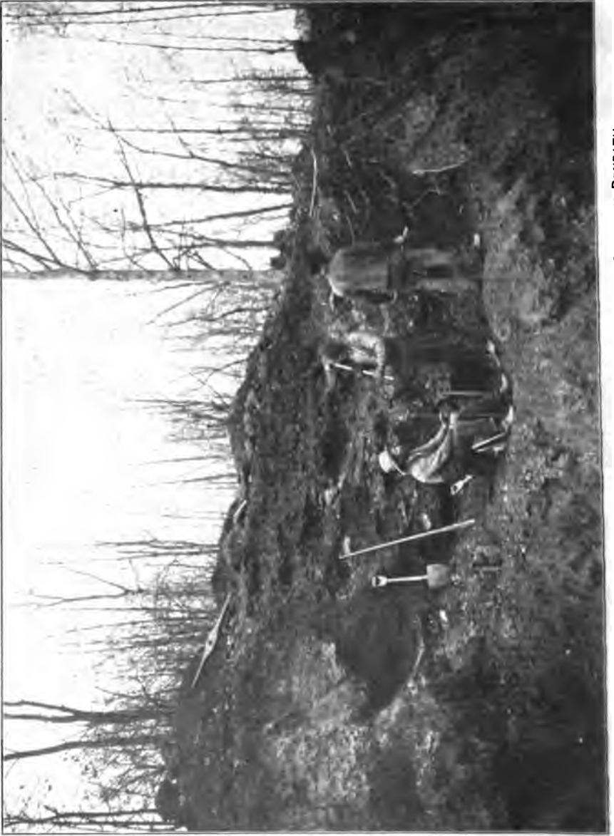
WORKMEN ON THE OUTER MARGIN OF THE MINE DISCOVER OPEN GALLERIES BENEATH.
