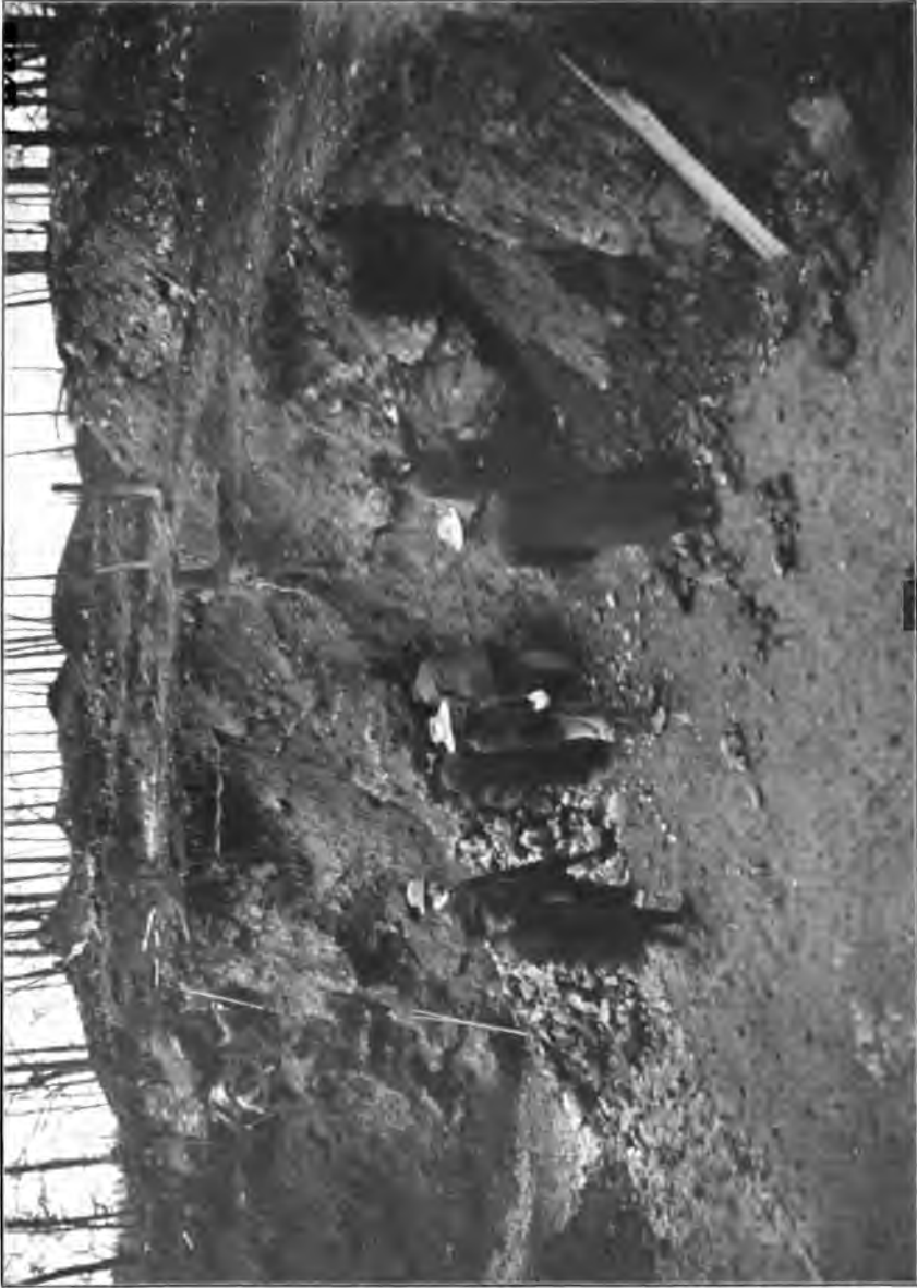
VIEW OF THE MINE WALL, SHOWING TRACES OF THE ANCIENT TUNNELS, EXTENDING DOWN THROUGH THE ORE BODY.
