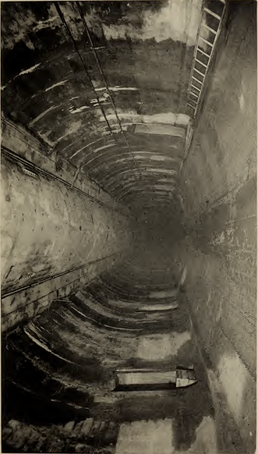
SECTION B OF THE EAST BOSTON TUNNEL,--SHOWING AIR DUCT IN ROOF. FEBRUARY 8, 1904.
