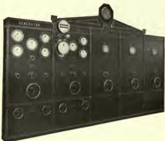
Switchboard for the power-station at Folkestone.
