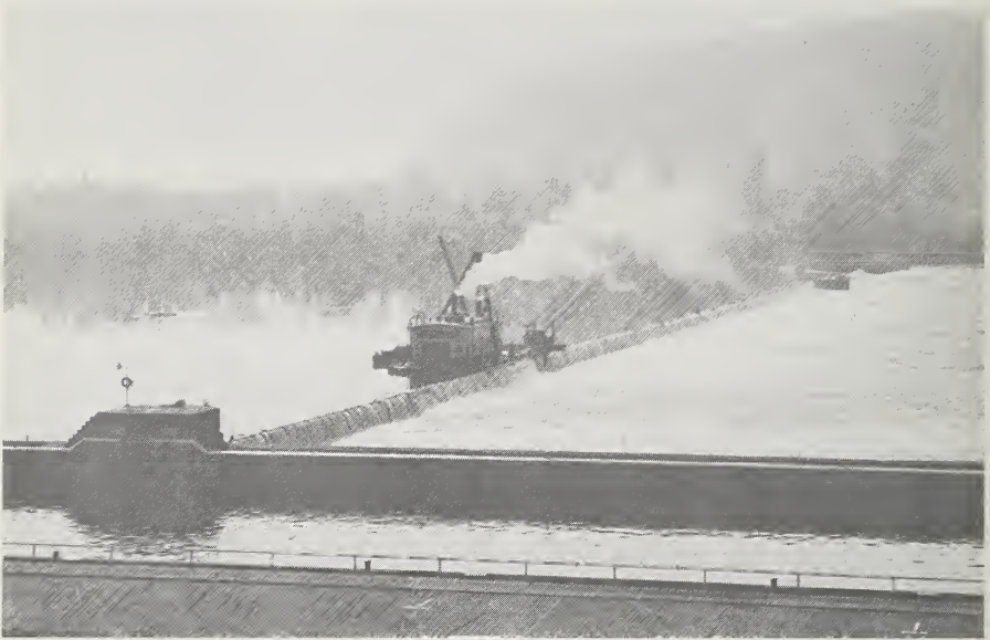
Co-op serves Ohio river dam at New Boston, Ind., opposite Fort Knox. Canal (foreground) permits ship and barge navigation down the Ohio to Cairo.
