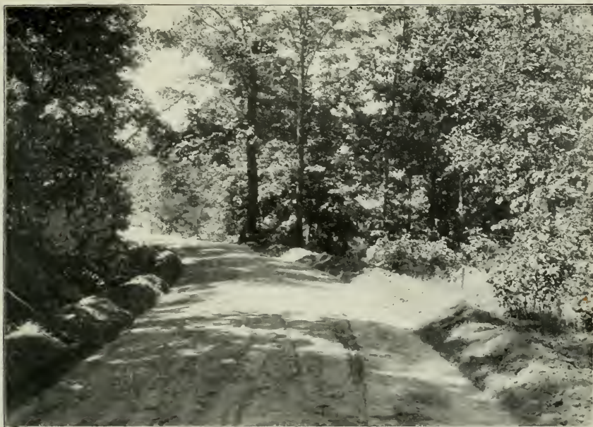
FIG. 1.—THE ROLLED FOUNDATION OF AN OBJECT-LESSON ROAD BUILT AT HOT SPRINGS, VA., UNDER THE AUSPICES OF THE OFFICE OF PUBLIC ROAD INQUIRIES OF THE DEPARTMENT OF AGRICULTURE.
